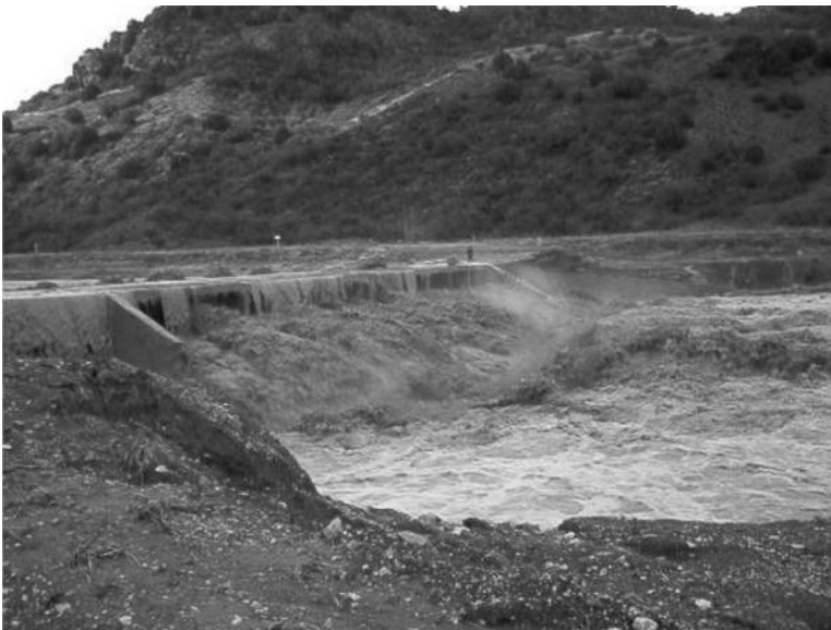
FIGURE 14.3 Concrete dike near Loveh Village is washed away.
