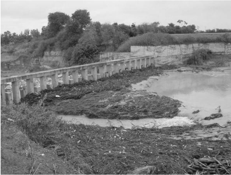
FIGURE 14.2 Destruction of Kordkoy Bridge due to flood.
