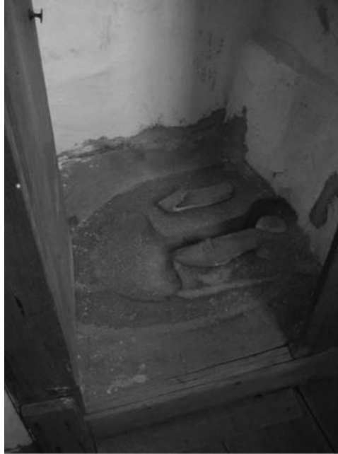
FIGURE 9.40 Squat toilet in mansion at Yürükköy, Anatolia. (Courtesy of E. Kanetaki.)
