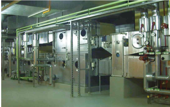
Fig. 3–49 Conventional climate control room
