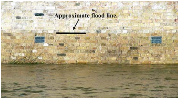
Figure 2. For some riverside properties, sandbags could not protect openings, such as those in the photograph (Cambridge, England, 2001)
