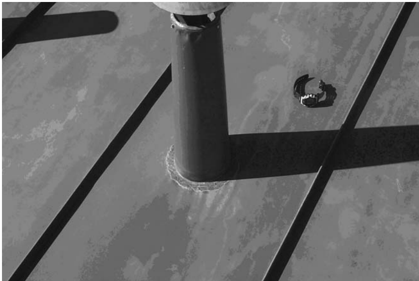
Fig. 10.2. Detail of roof construction: The antimony-free solder sealing material used to seal the chimneys on the roof.
