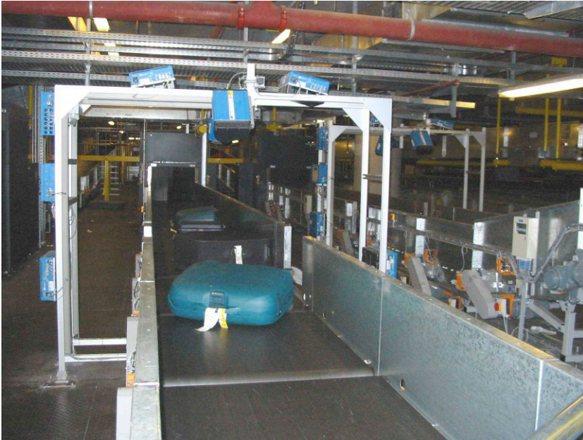
Fig. 3.1 The luggage handling system at Brussels Airport, Zaventem, Belgium
