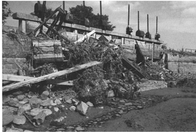
Photo 7. Dam Dolejsi—blocked protected old spillway (8 pcs).
