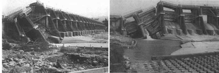
Figure 2. Shih-Kang weir in Taiwan, destroyed by fault movement during the September 21, 1999 Chi-Chi earthquake (courtesy Dr. R.Charlwood).
