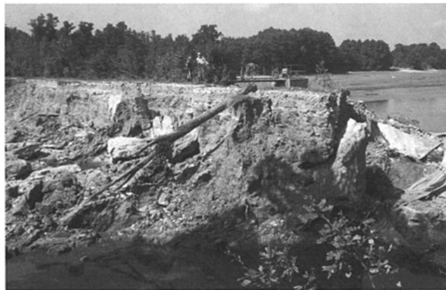
Photo 4. Dam Podhajsky—total gash with eroded downstream side.
