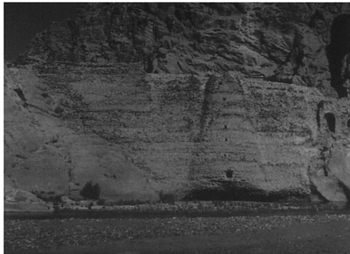
Figure 7. Ruins of Saveh dam, which was demolished in the meantime.
