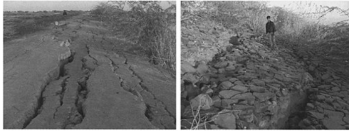
Figure 1. Earth dams damaged by the January 26, 2001 Bhuj earthquake, Gujarat, India (courtesy Prof. S.K.Jain).
