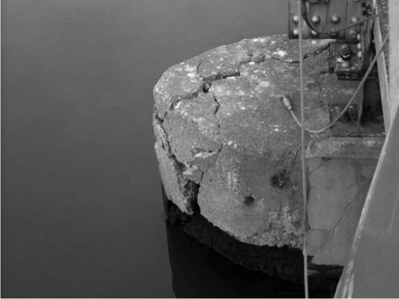
FIGURE 8-7. Backlog of Maintenance Example: Deteriorated Concrete on Dam Pier. Courtesy of U.S. Army Corps of Engineers.
