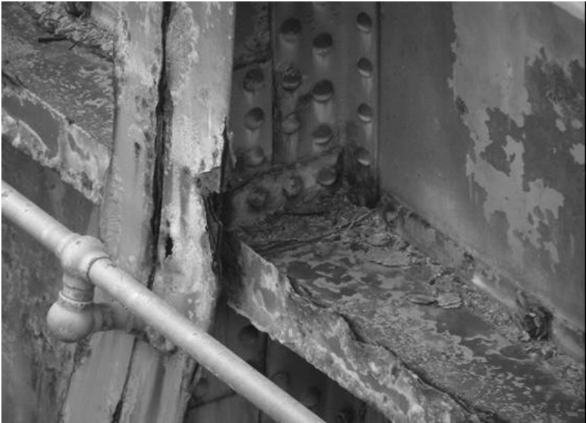
FIGURE 8-8. Backlog of Maintenance Example: Deteriorating Dam Gate. Courtesy of U.S. Army Corps of Engineers.
