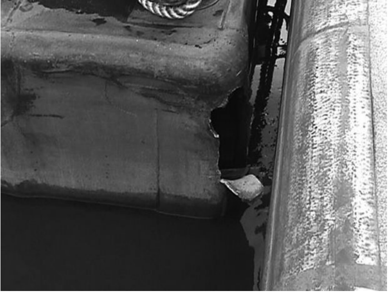
FIGURE 8-5. Backlog of Maintenance Example: Barge Damaged—Hit Wall Armor Plating. Courtesy of U.S. Army Corps of Engineers.
