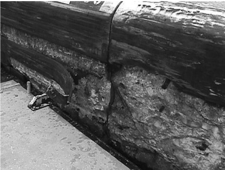
FIGURE 8-4. Backlog of Maintenance Example: Damaged Wall Armor Plating. Courtesy of U.S. Army Corps of Engineers.
