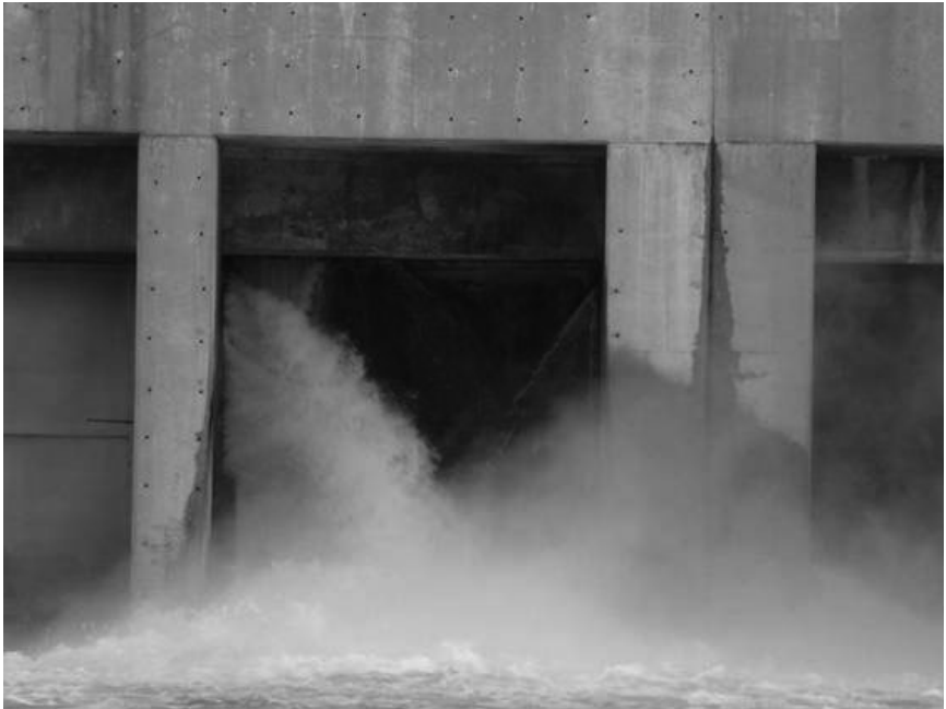
FIGURE 8-6. Backlog of Maintenance Example: Leaking Dam Head Gate. Courtesy of U.S. Army Corps of Engineers.
