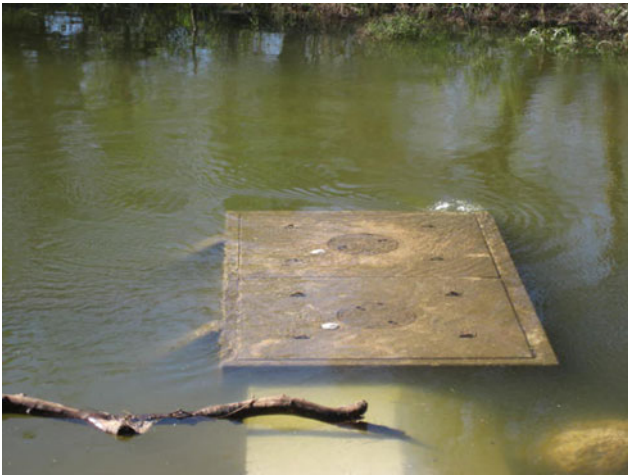
Fig. 11 Photograph of the top of the BMP about 8 h past the peak storm pulse on October 27, 2009, with a whirlpool near the corner of the vault due to water entering the original valve
