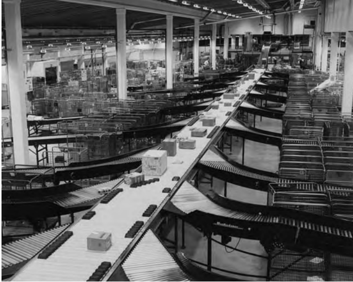
FIGURE 11.1 Conveyor system. (Courtesy of Vanderlande Industries, The Netherlands. With permission.)
