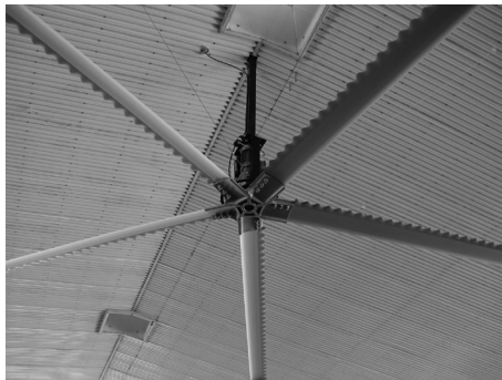
Figure 10.5 Industrial fan with WhalePower blades.
