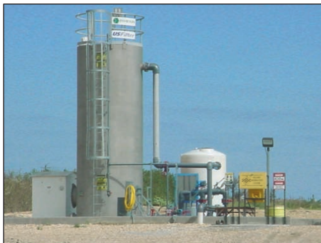
Figure 9.3 Ex situ bioreactor at NWIRP McGregor, McGregor, Texas (Photo courtesy of NAVFAC Southeast)
