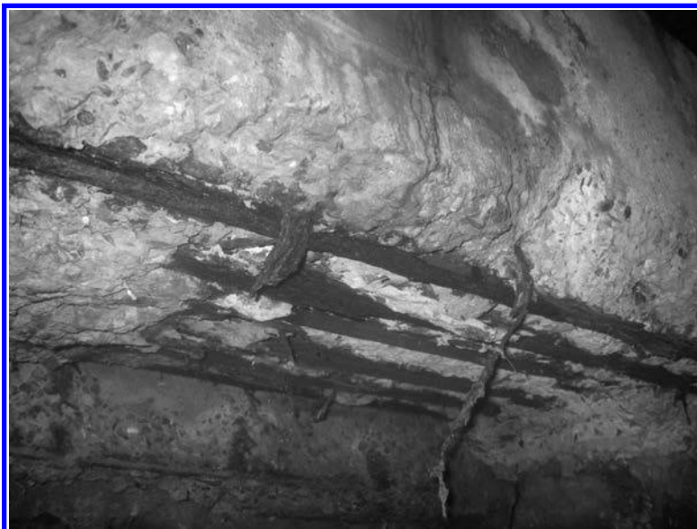
FIGURE 5.5 Corrosion of reinforcing bars in the bottom of a reinforced concrete bridge.
