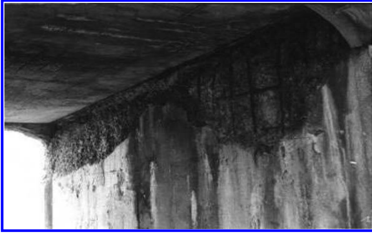
FIGURE 5.6 Corrosion of reinforcing bars in the abutment of a reinforced concrete bridge.
