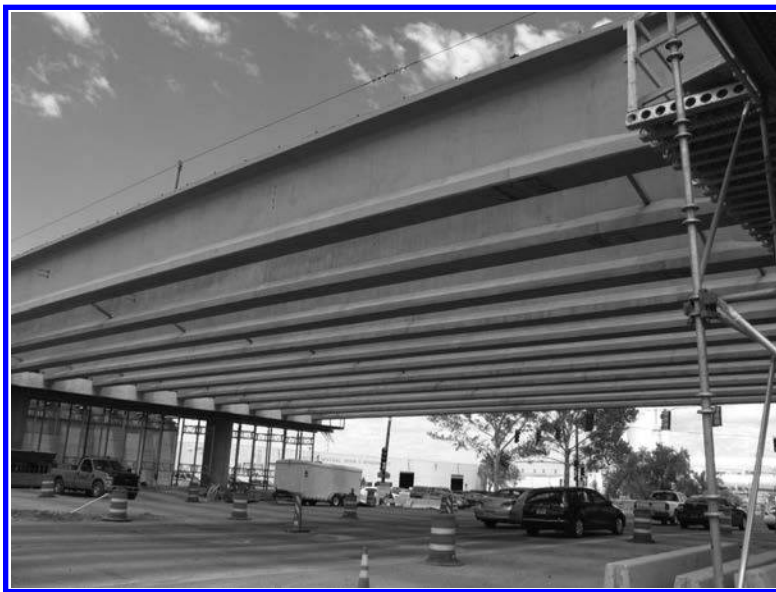
FIGURE 5.118 A precast, prestressed concrete girder bridge over Jefferson Street, Albuquerque, NM, under construction (August 2014). This superstructure consists of 11 AASHTO-PCI bulb-T girders.
