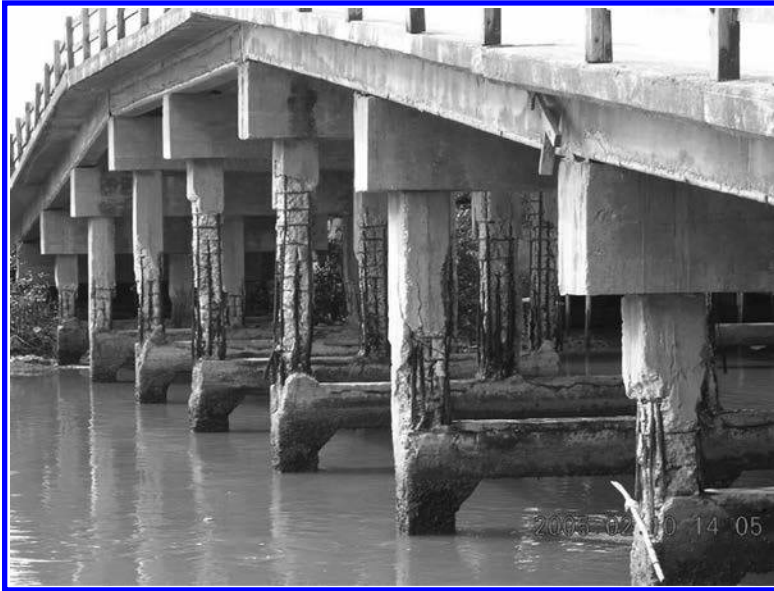
FIGURE 5.8 Corrosion of reinforcing bars in the bents of a reinforced concrete bridge.
