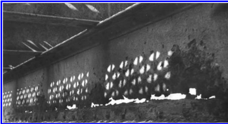
FIGURE 6.13 An extremely corroded floor beam in a steel through truss bridge of Figure 6.12 (inspected by the author). Note that a bottom portion of the corroded web has crumbled and disappeared resulting in loss of cross-sectional area and load-carrying capacity.
