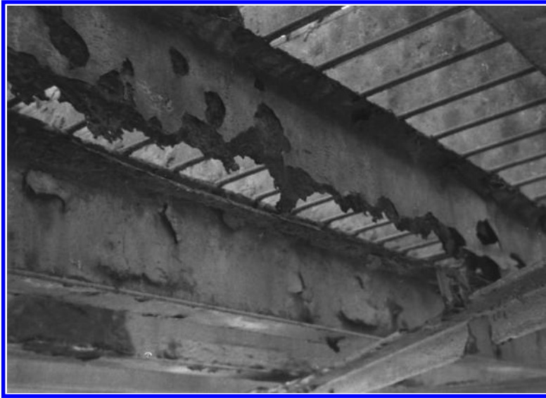
FIGURE 6.12 An extremely corroded steel stringer supporting an open steel deck of a steel through-truss bridge (inspected by the author). The corroded web of the stringer is clearly visible; a portion of the web has crumbled and disappeared resulting in loss of cross-sectional area and load-carrying capacity.
