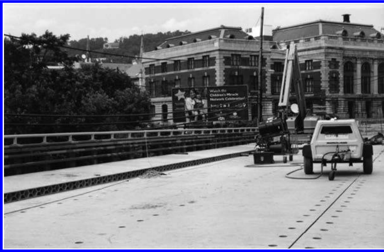
FIGURE 2.23 An FRP highway bridge superstructure deck system built from pultruded units shown in Figure 2.22 . These units are clearly visible underneath the sidewalk on the left. (Market Street Bridge, Wheeling, West Virginia, nearing completion.) (Photo by author.)
