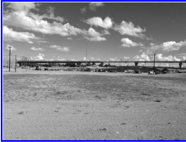
FIGURE 6.6 A nine-span, curved, prestressed concrete girder and steel plate girder combination highway bridge over Interstate-25 under construction in Albuquerque, New Mexico (September 2014). The photo shows six spans beginning at the west end of the bridge. The three west-end approach spans and the south-end approach span are simply supported by precast, prestressed concrete bulb-T girders. The intermediate five spans consist of continuous, curved steel plate girders. (See details in Figure 6.7a–c .)
