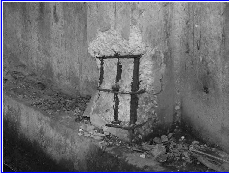
FIGURE 5.7 Corrosion of reinforcing bars in the pier of a reinforced concrete bridge.
