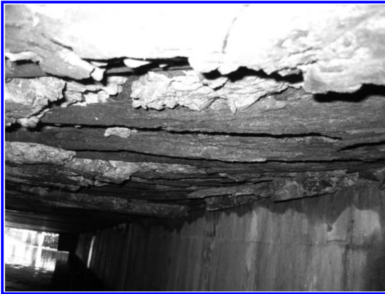
FIGURE 1.8 Severe and extensive corrosion of tensile reinforcing bars and spalling of concrete at the bottom of a deck slab.
