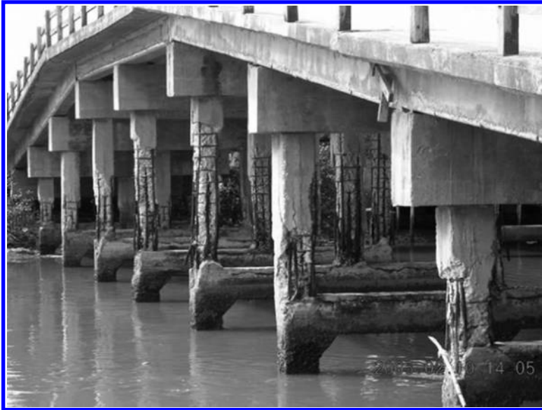
FIGURE 1.9 Severe corrosion of reinforcing bars and spalling of concrete in the bents of a reinforced concrete bridge.
