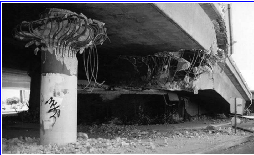
FIGURE 3.90 Complete collapse of bridge carrying Interstate 10 (Santa Monica Freeway) in Los Angeles during the 1994 Northridge earthquake.
