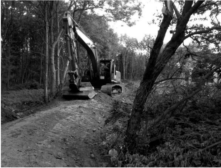
FIGURE 6.9 Establishment of embankment at Godsparken in Greve. (From DANVA, Urban Climate Change [Original title: En kagebog for analyser af klimaændringers effekter på oversvømmelser i byer], 2011.)
