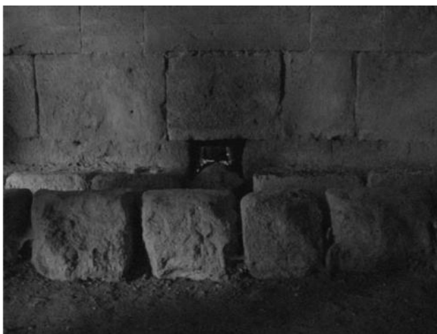
FIGURE 9.39 Latrines placed one next to the other and the sewage hole in the Aksaray Sultan Han. (Courtesy of G. Antoniou.)
