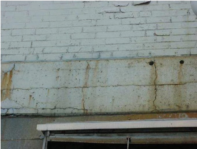
Figure 6.3: Concrete beam cracking from corrosion of reinforcing steel.
