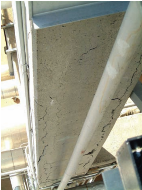
Figure 6.4: Concrete column cracking and spalling.
