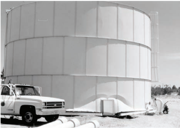
Figure 7.3: Above: Tank Wall Failure at Tank Manhole Access Bighorn Desert View Water Agency, Water Storage Tank, Landers, CA
