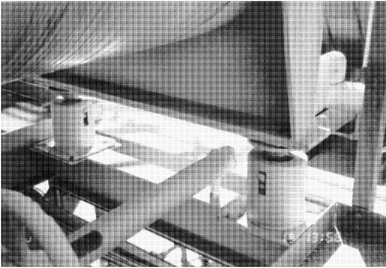
Figure 6.10: Load cells are commonly used in the support for vessels. These may lack capability of resisting lateral loads and should be carefully examined.
