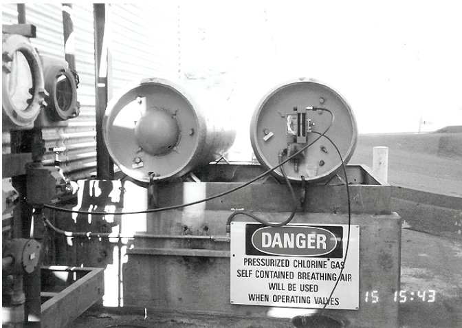
Figure 6.13: Cylinders that are removed when empty often sit unrestrained on vertical saddle shaped supports. In this photo, a simple hold-down bolt prevents motion while the cylinder is in use. The presence of a mechanism like this can be judged to reasonably prevent overturning or sliding of the cylinder.
