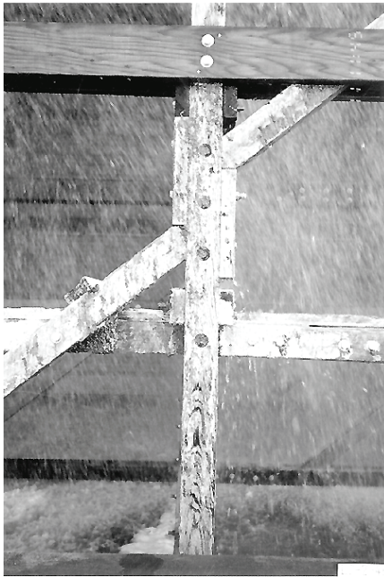
Figure 6.18: Eccentrically loaded connection in a wood cooling tower. The cross member above is a retrofit.
