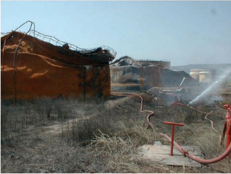
Figure 7.6: Damaged Tanks Due to Fire After Earthquake, 1999 Izmit, Turkey Earthquake
