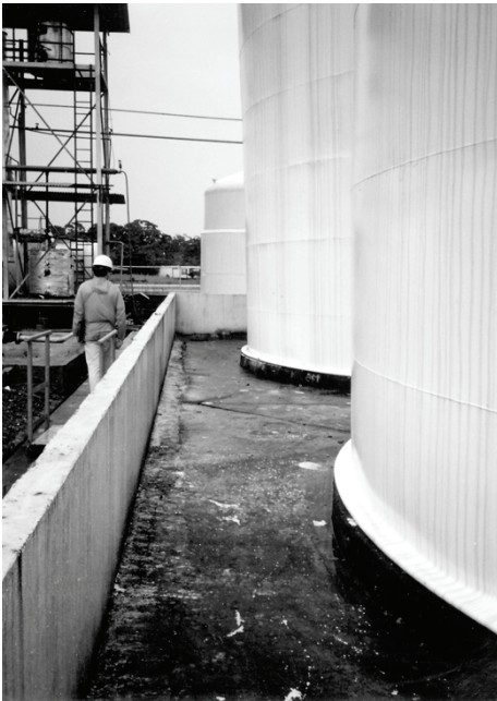
Figure 7.5: Above: Damaged Roof, Seals, and Sloshing of Oil over Tank Walls, RECOPE Oil Refinery, Costa Rica
