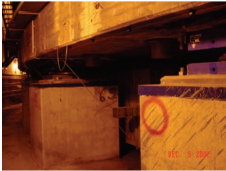
Figure 5.5: Base Isolated LNG Tank, Greece
