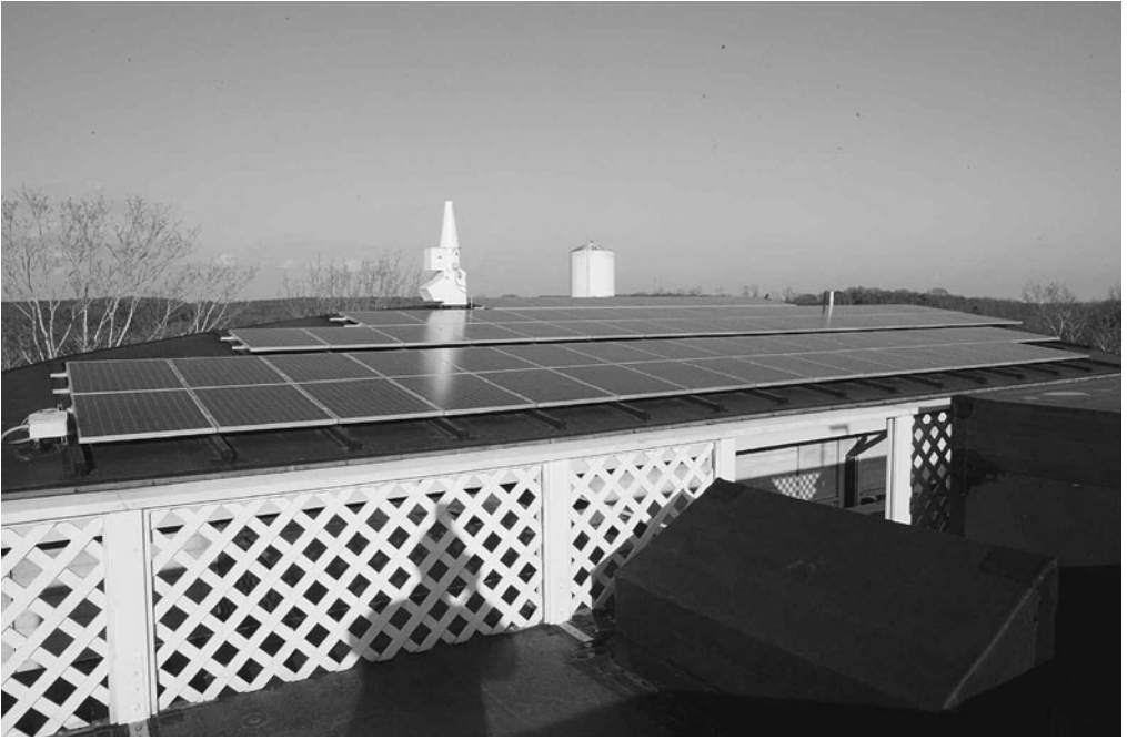
Figure 3.5 The exhaust for the hood in the chemical laboratory had to be installed after the rooftop electrical panels. The tank in the background to the right is a large town-owned water tank on a rise to the northward behind the building.
