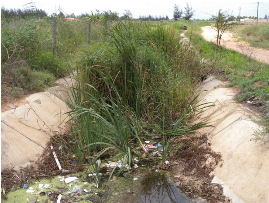
Fig. 13.5 Maputo, KaMavota district, 3 Nov. 2011. Stormwater drainage along Dona Alicia Street with efficiency compromised by vegetation (Tiepolo 2011)
