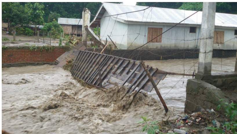
Fig. 6 A footbridge damaged by Lanva River in July 2015
