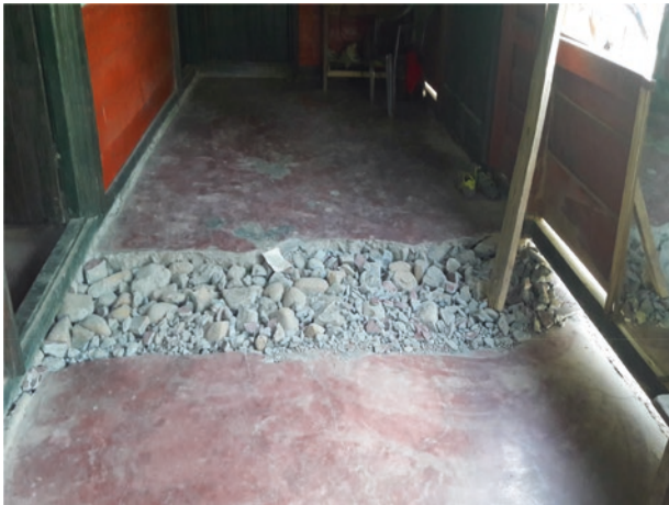
Fig. 6 An earthquake affected house in Noney
