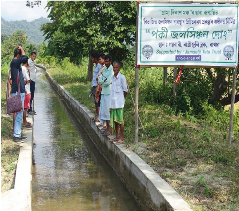
Fig. 2 ‘Diversion Based Irrigation’ canals constructed by Gramya Vikash Mancha (GVM) with the labour participation of the villagers in Nagriju Block, Baksa district ( Source Photograph taken by the author during fieldwork)
