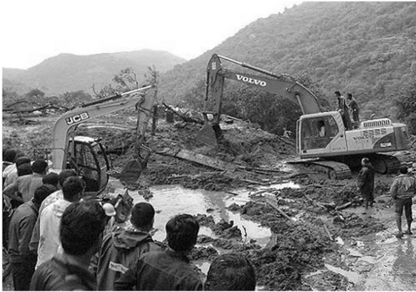
Fig. 2 Landslide in village of Malin on 30 July 2014 in Pune, Maharashtra
