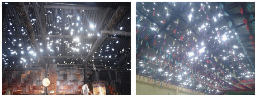
Fig. 1 Hail damaged galvanised iron sheet roofings
