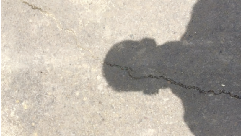
Fig. 2 Cracks in the dam
