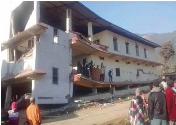
Fig. 4 Collapsed women market in Saikul
