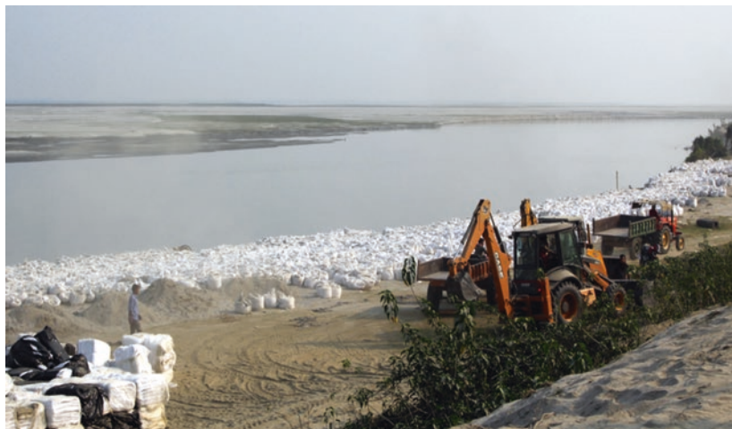
Fig. 4 The ongoing construction of the new embankment in Matmora where geotube technology is being used for the first time in India
