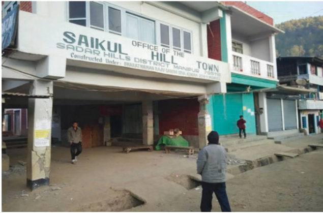
Fig. 5 Pillars of the office of the Saikul Hill Town developing cracks after 4th January Manipur earthquake
