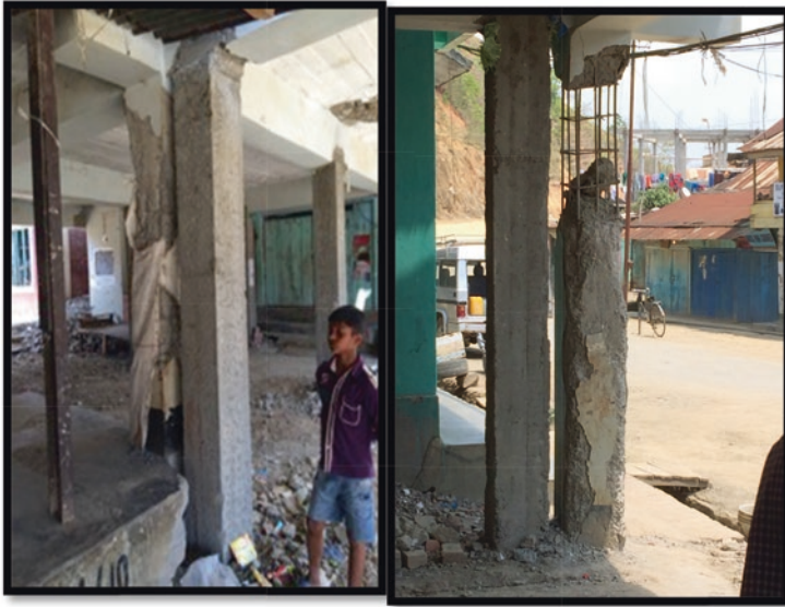
Fig. 6 Propping damaged RCC structures by newly constructed columns not connected to the beam above
