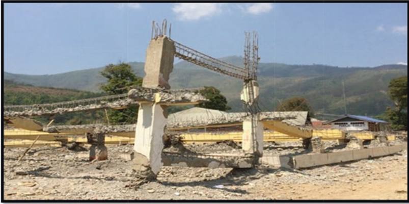
Fig. 3 Collapsed frame of a soft-storeyed RCC structure (women vendors' market) in Saikul
