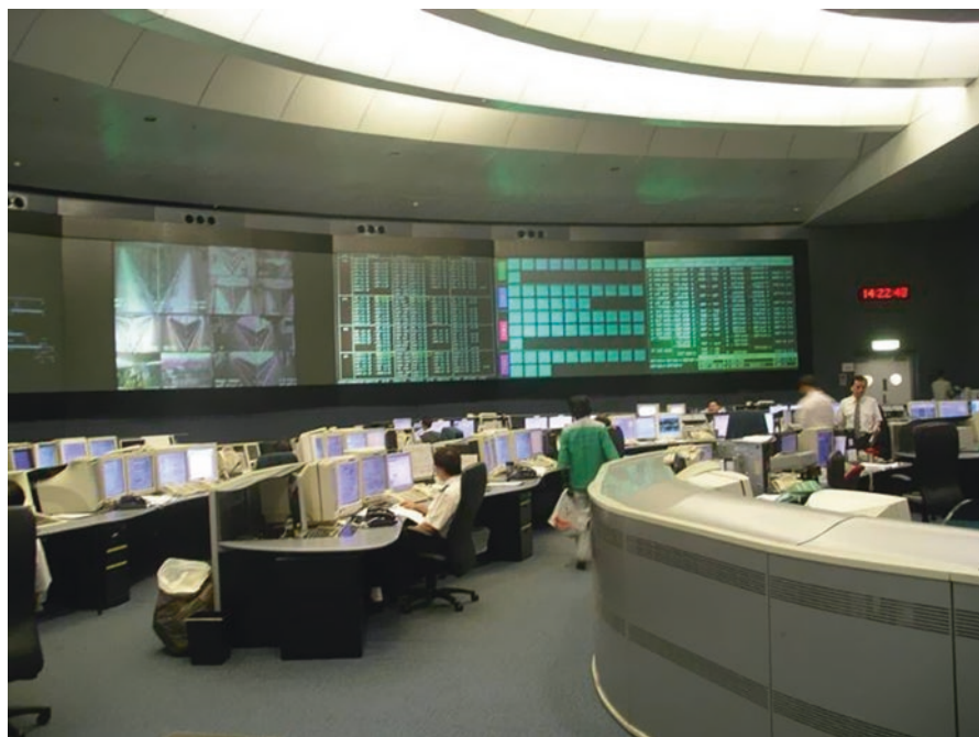
Plate 6.2 The control centre of the automatic train operation system of the MTR in Tsing Yi (青衣) station (photo taken by the author in 2007)
