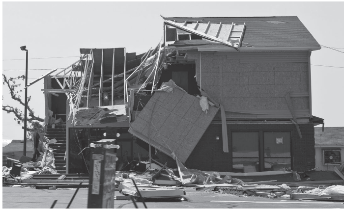
Photo 2.3: The connection of this roof was unable to resist the large uplift due to heavy winds. The left side roof was carried away entirely, while the right side began to peel off the top of the structure. Much like uplift, the outward pressure on the side walls has torn off the siding. The ASCE design wind pressure expression indicates the pressure direction so engineers can apply the resulting forces on building roofs and wall cladding in order to properly design their connections.
