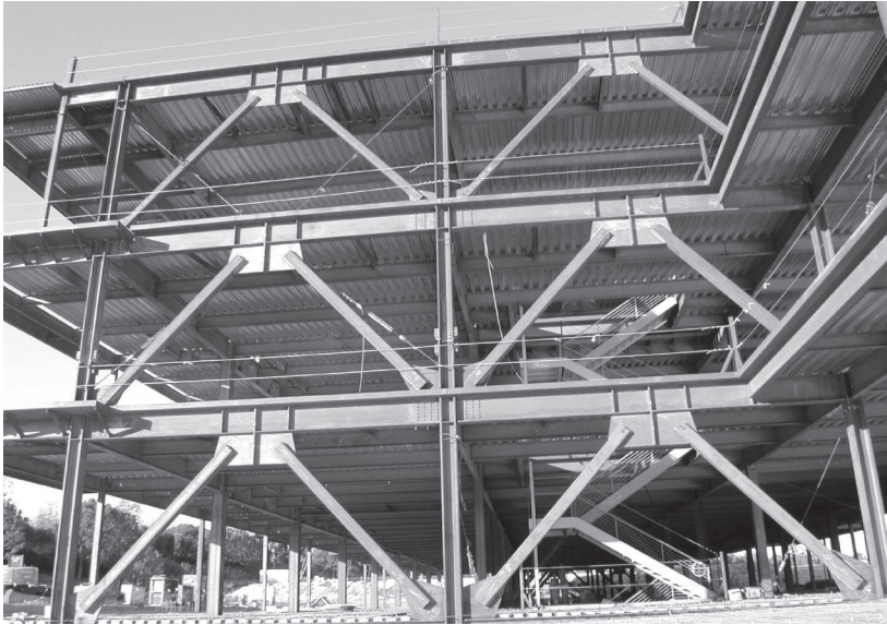
Photo 2.1: The diagonal-bracing, together with the attached columns and horizontal floor beams in the plane of the bracing, forms a deep continuous, vertical truss that extends the full height of the building (from foundation to roof) and produces a stiff, lightweight structural element for transmitting lateral wind and earthquake forces into the foundation.
