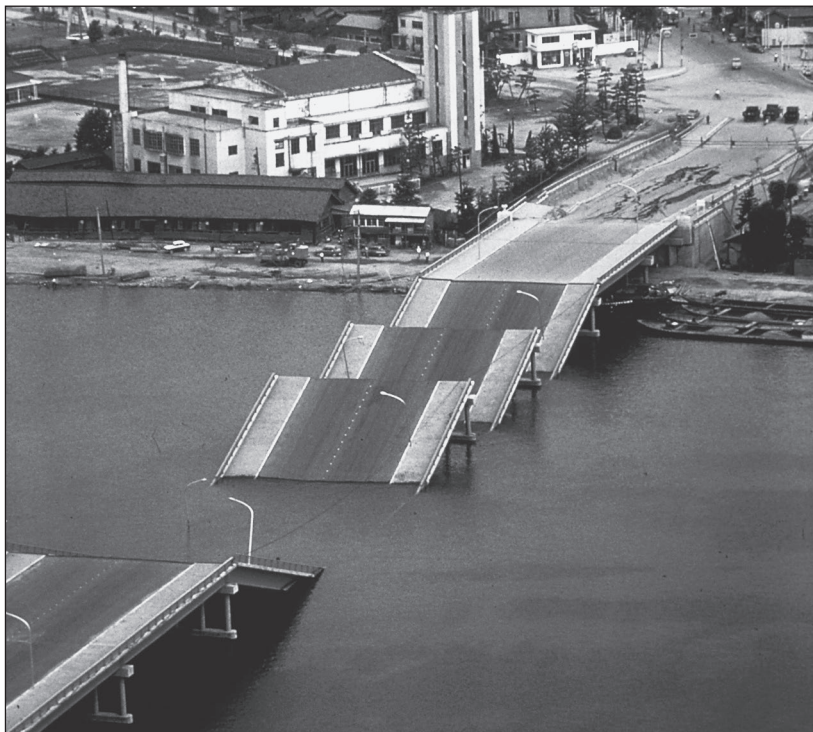
Photo 3.3: An example of the collapse of a bridge composed of simply supported beams during the 1964 Nigata earthquake is shown here.
