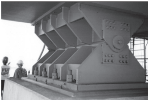
Photo 3.1: Pin support for the 2.1-mile long steel box girder San Diego-Coronado Bridge.
