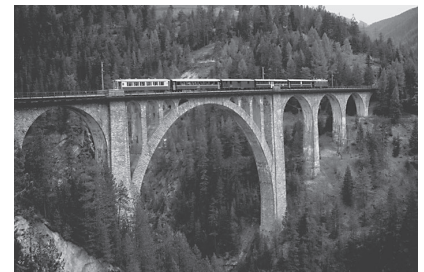
Photo 6.3: Railroad bridge (1909) over the Landwasser Gorge, near Wiesen, Switzerland. Masonry construction. The main arch is parabolic, has a span of 55 m and a rise of 33 m. The bridge is narrow as the railway is single-track. The arch ribs are a mere 4.8 m at the crown, tapering to 6 m at the supports. Courtesy of the Godden Collection, NISEE, University of California, Berkeley
