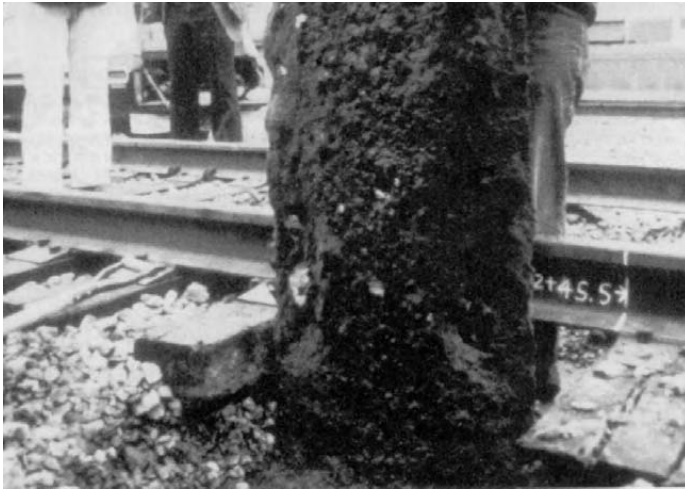
Figure 5.22 Abrasion failures of geotextiles placed too close to the track structures (after Raymond, 1982).
