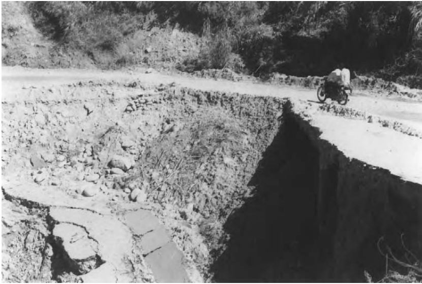
Figure 4.37 A severe landslide causing inconvenience to traffic movement (after Shukla and Baishya, 1998).
