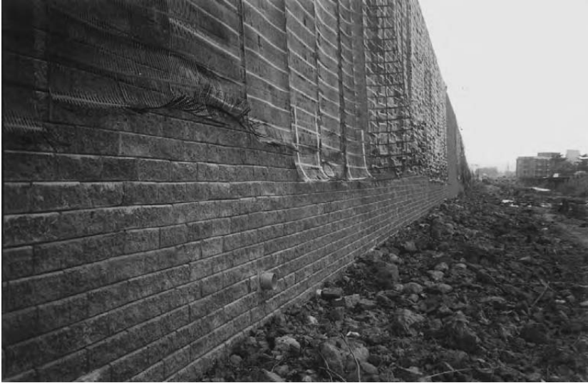
Figure 9.3 A portion of retaining wall on the Mumbai–Pune Expressway (Panvel Bypass–Package I), India during its construction stage (courtesy of Netlon India, 2001).
