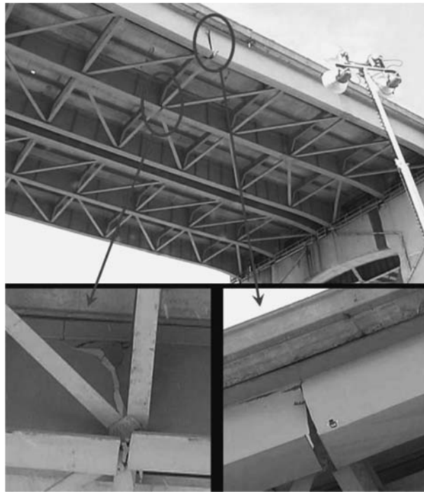
Figure 15 Hoan Bridge fracture.
