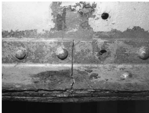
Figure 19 Fatigue crack in heavily corroded flange angle and web plate.
