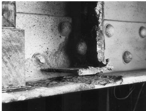
Figure 18 Corrosion notch in flange angle of riveted member under a diaphragm.
