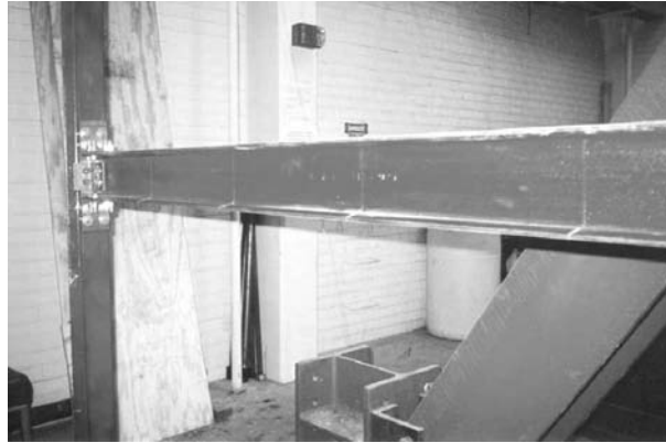
Figure 11 Four cracks in a beam.
