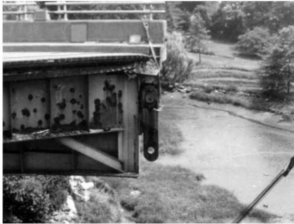
Figure 20 Collapse of suspended span of Mianus River Bridge, Connecticut.
