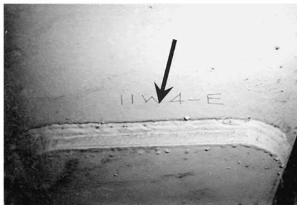
Figure 5 Yellow Mill Pond Bridge: fatigue crack at the end of cover plate.
