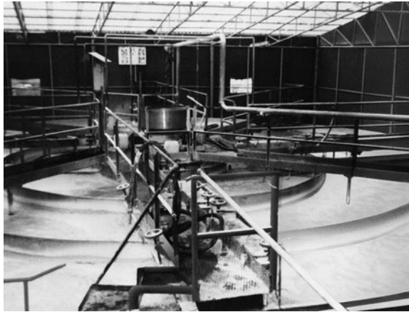
Fig. 12.2. An installation with a 40 ft-diameter IAF cell.
