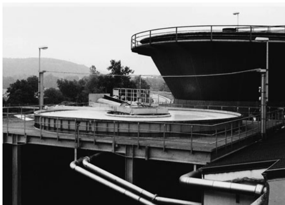
Fig. 12.4. 55 ft-diameter DAF clarifier.
