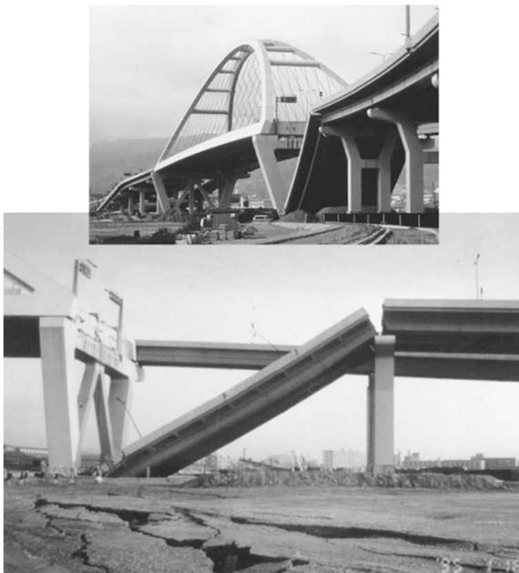
Fig. 16.3 A bridge approach span collapse during the 7.2 magnitude 1995 Kobe earthquake (photo courtesy of Kobe Collection, EERC Library, University of California, Berkeley)
