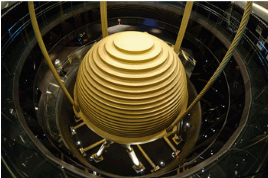
Fig. 1.23 A 660 ton pendulum tuned mass damper system installed in the Taipei World Financial Center (with a height of 509.2 m) to mitigate the wind- and earthquake-induced responses of the building. The TMD hangs from the 92nd to the 88th floor
