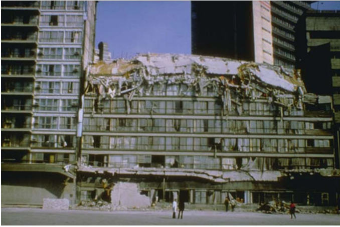
Fig. 3.4 Collapse of top stories of Hotel Continental in Mexico City during the 8.1 magnitude Mexico City earthquake of 1985
