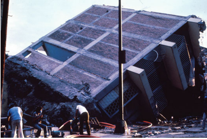
Fig. 1.3 An eight-story building was broken into two during the 8.1 magnitude of earthquake occurred in Mexico City in 1985
