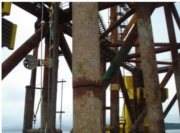
Fig. 1.11 A primary structural member of an offshore jacket structure breaks due to the repeated wave loading. The photo was taken after the jacket structure was decommissioned and transported onshore
