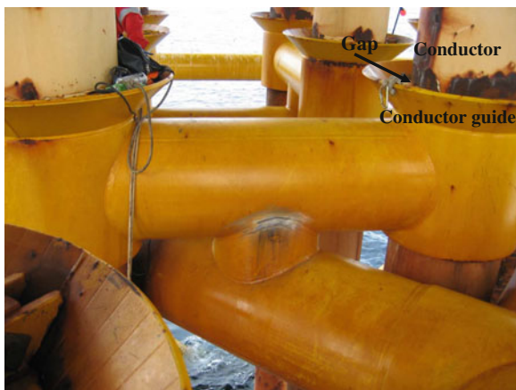
Fig. 15.19 Conductor and conductor guide installed on an offshore platform (courtesy of Aker Solutions)
