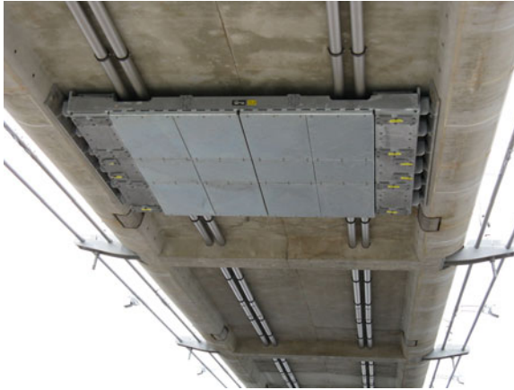
Fig. 2.7 TMDs installed under the bridge deck of the Infinity Bridge (photo by John Yeadon)
