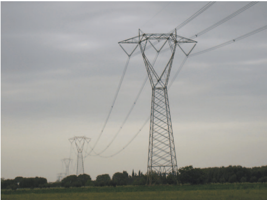
Fig. 9 High voltage (380 kV) overhead power line. (authors' image)
