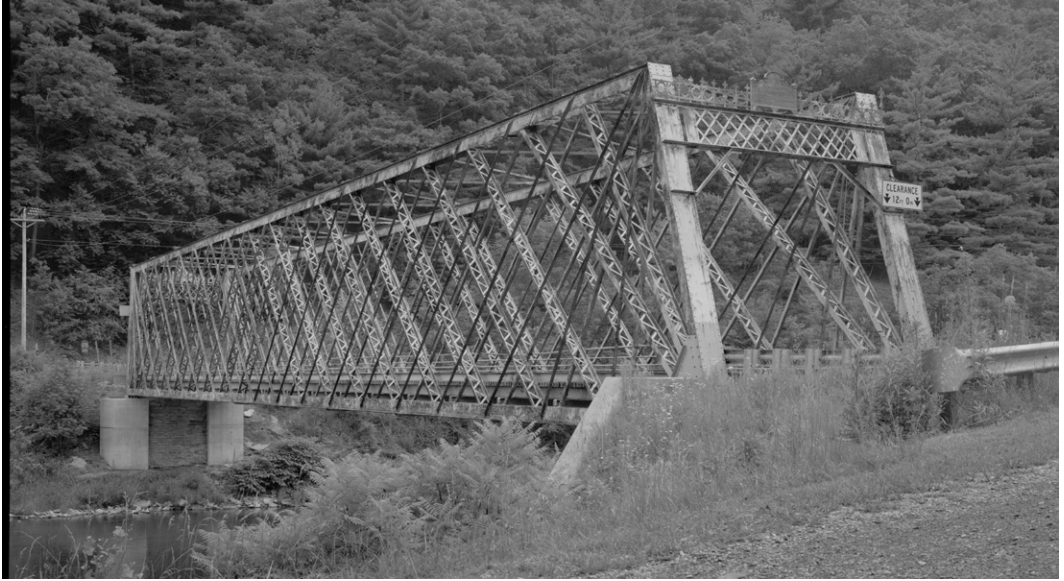
Figure 1-8. Upper Bridge at Slate Run, spanning Pine Creek at State Route 414, Slate Run, Lycoming County, PA. Quintuple Warren truss bridge (HAER PA,41-SLARU.V,1-3). Source: Photograph by Joseph Eliot.
