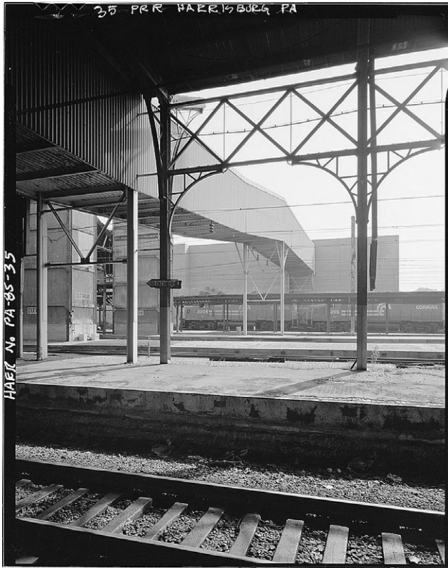
Figure 10-5. Portals at Harrisburg, PA, train station (HAER PA,22-HARBU,23-25). Source: Photograph by F. Harlan Hambright.
