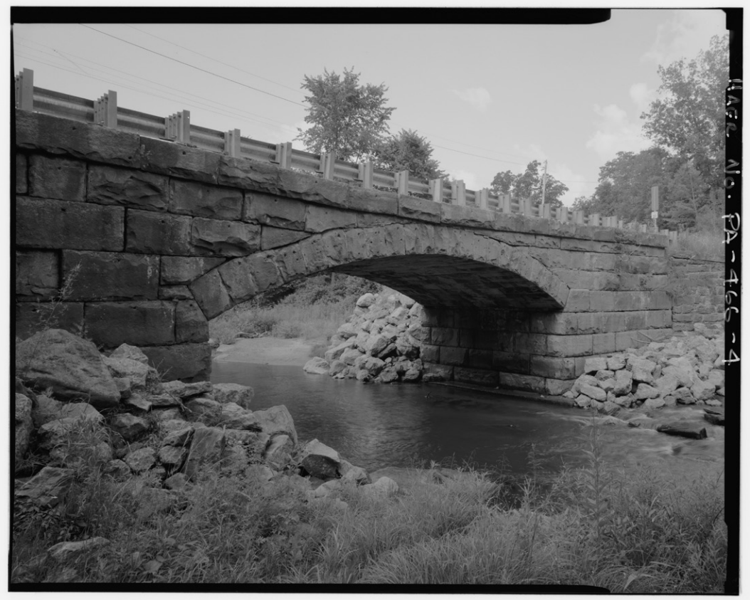
Figure 2-1. Pithole stone arch bridge, spanning Pithole Creek at Eagle Rock Road (State Route 1004), Pithole City, Venango County, PA (HAER PA,61-PIT,1-).
