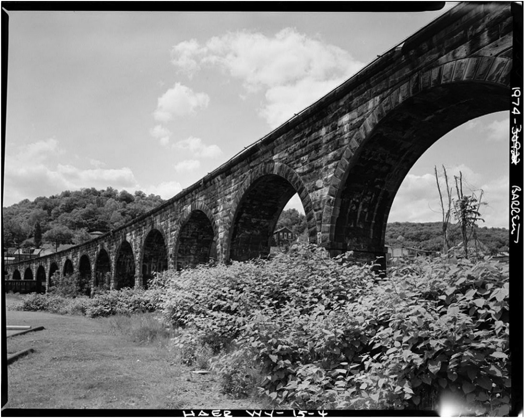
Figure 6-1. Example of a railroad masonry arch bridge. Baltimore and Ohio Railroad, Benwood Bridge, Marshall County, WV (HAER WVA, 26-BEN, 1–4).
