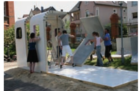
fig. 10 | Installation of an inside layer of textile-reinforced concrete (inlaid with capillary pipes) to seal the shape
