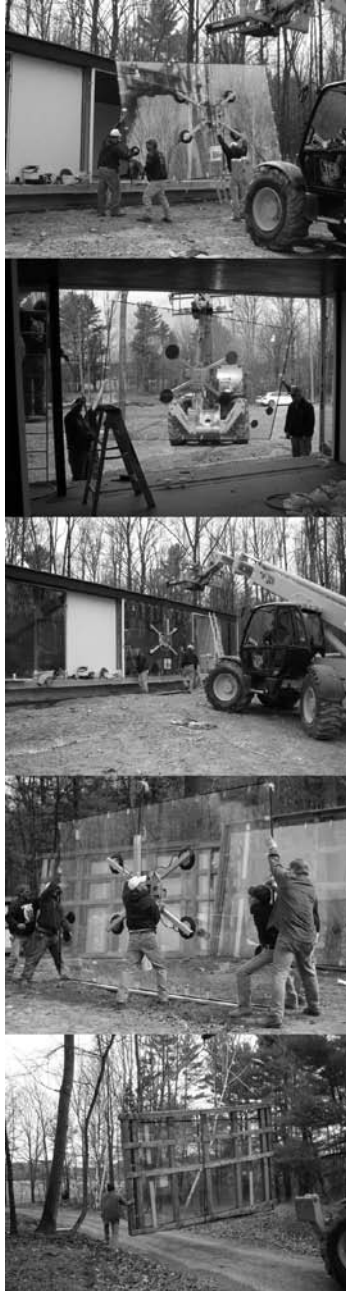
fig. 3 | IGU installation maintains vertical integrity of assembled unit, as compared with horizontal production of float glass
