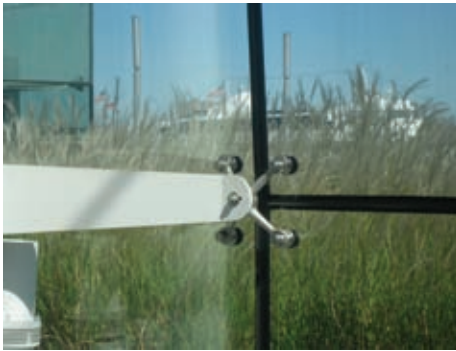
fig. 4 | Detail of glass connection, West Midtown Ferry Terminal, William Nicholas Bodouva + Associates, New York, N.Y.
