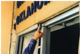
fig. 1 | Storefront glazing fracture in Oklahoma City bombing
