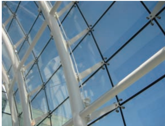
fig. 5 | Detail of glass connection at curve, West Midtown Ferry Terminal, William Nicholas Bodouva + Associates, New York, N.Y.
