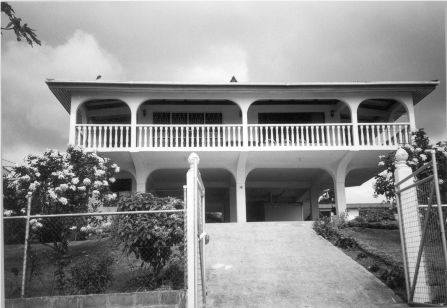
Figure 13.7 Highly asymmetrical reinforced concrete house in Suva, Fiji, with weak bottom storey, which could be cheaply retrofitted with bracing to prevent collapse
