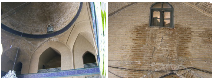
Figure 5: Water damage after earthquake.
