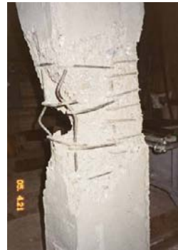
Figure 6: Virgin specimen without confinement.
