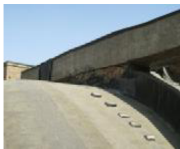
(b) Damage in Arch keystone
