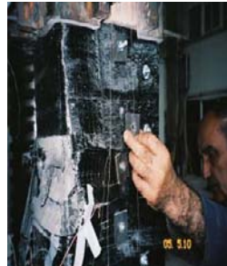
Figure 8: Failure of anchor bolt.
