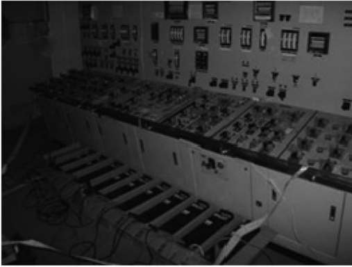
Figure 6. Temporary batteries were connected to instruments to power them.
