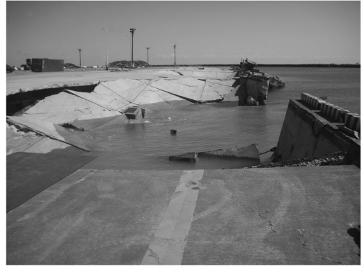
Photograph 1. Combined Damage by Earthquake and Tsunami at Port of Soma (Taken by Tohoku Regional Bureau of MLIT).
