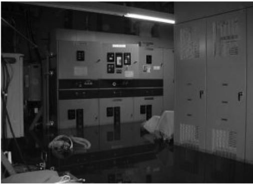
Figure 13. Flooded switch gear in unit 6.
