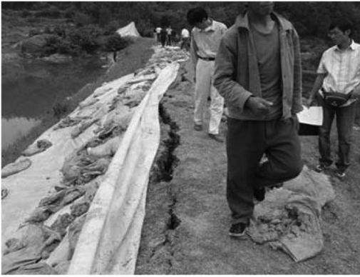
Figure 4. Cracks on Shidaojiao reservoir dam in Guanyuan City after Wenchuan earthquake.
