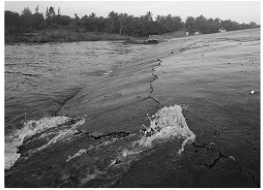
Figure 2. Cracks on Wanquanhe dam (Qionghai, Hainan Province).
