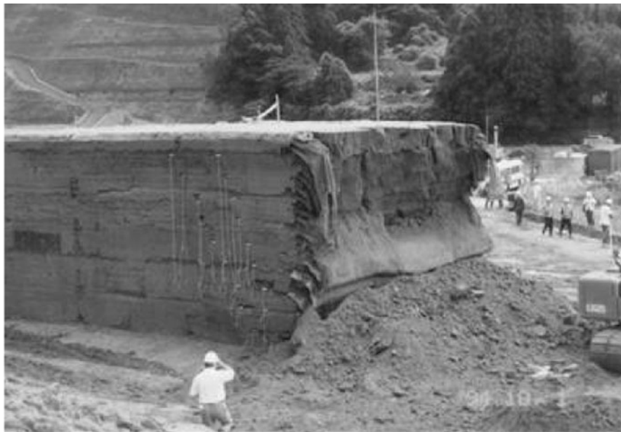
Fig. 7.5 Overhanging cliff (Step 6), collapsed completely
