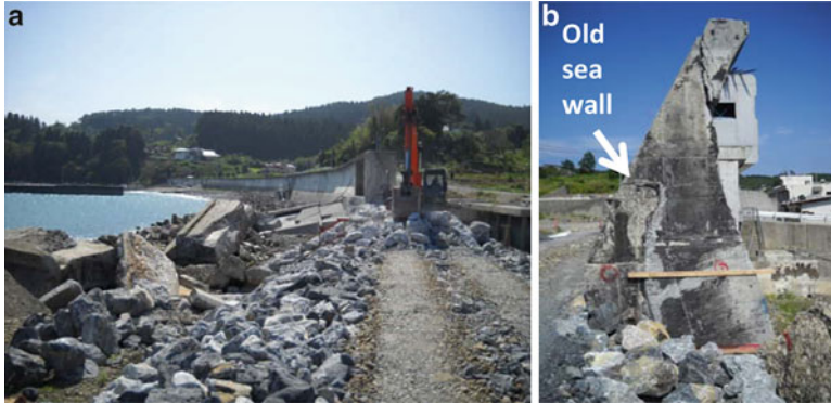
Fig. 2.11 Photos of seawalls with improvements prior to the tsunami. (a) Damaged sea walls in Ofunato City. (b) Evidence of improvements
