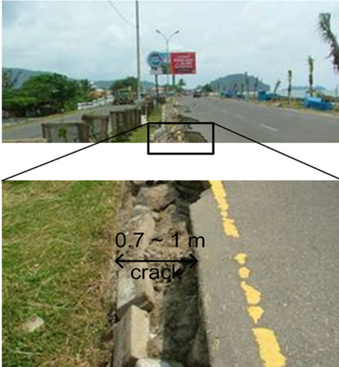
Fig. 4.7 Lateral spreading affecting the Seafront road (Jalan Samaudra) in Padang
