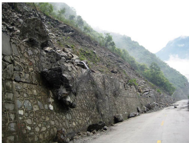
Fig. 5.6 Failure of a negative net at the Pubugou dam site
