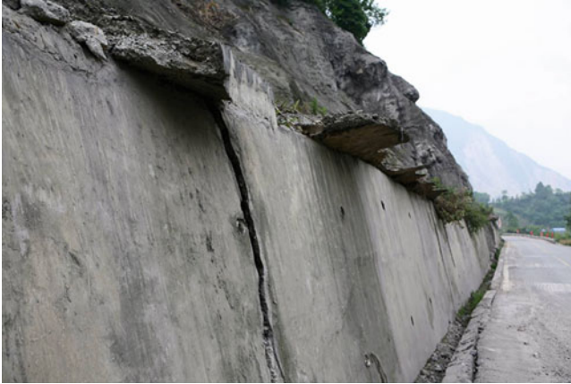
Fig. 5.7 Failure of shotcrete along highway G213
