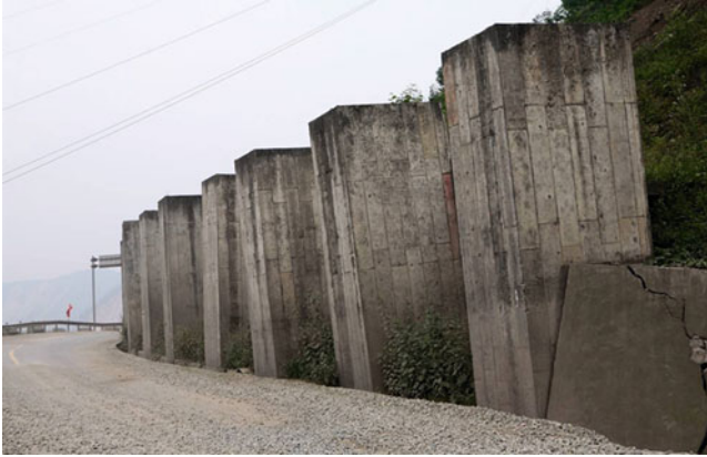
Fig. 5.10 Piles in Xuankou town along highway G213
