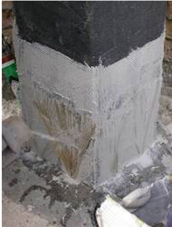
Fig. 6.32 Flexural strengthening at the footing joint of a RC column using steel spikes wrapped with a FRP jacket (Prota et al. 2005)
