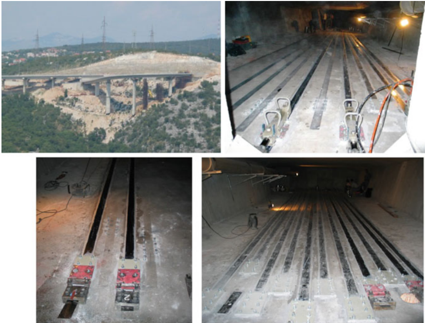
Fig. 7.25 Bridge box girder strengthening, Rijeka (Croatia), courtesy of S&P Clever Reinforcement AG
