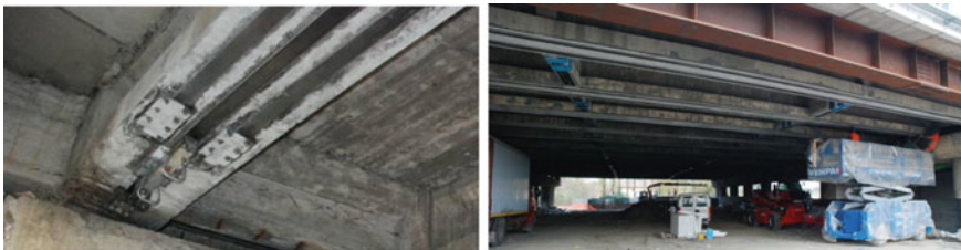
Fig. 7.31 Strengthening of the girders of the Battiferro-Navile viaduct (A14 Highway Bologna-Taranto, Italy), courtesy of Prof. Dr. Carlo Pellegrino and Giorgio Giacomini
