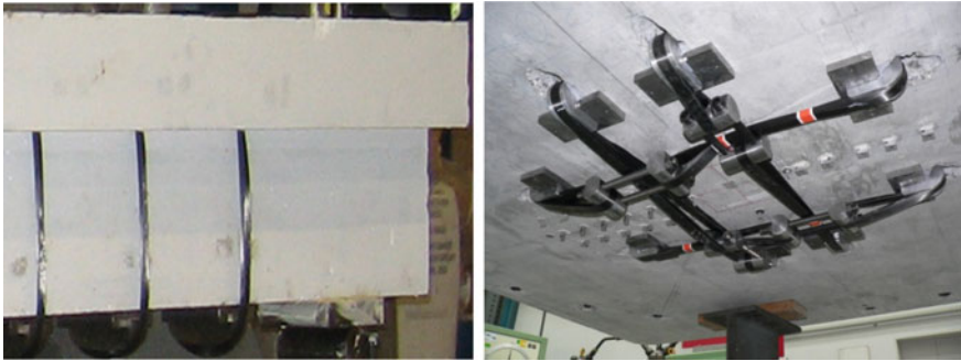
Fig. 7.19 CFRP strap strengthening of a T-beam (©University of Cambridge) and a flat slab (courtesy of Dr. A.U. Winistörfer)
