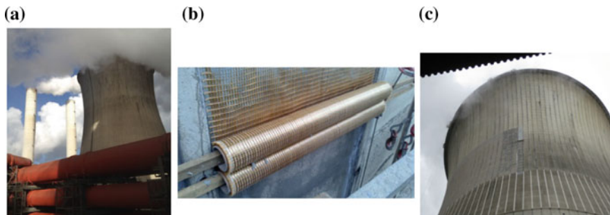
Fig. 9.1. Structural retrofitting of cooling towers with PBO-FRCM (by Ruredil): a Power plant cooling tower. b and c application of the FRCM composite
