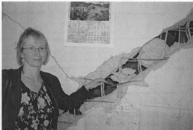
Figure 13.27 Shear failure of a reinforced concrete shear wall in the May 2003 Boumerdes, Algeria earthquake; note the fractured horizontal reinforcement.
