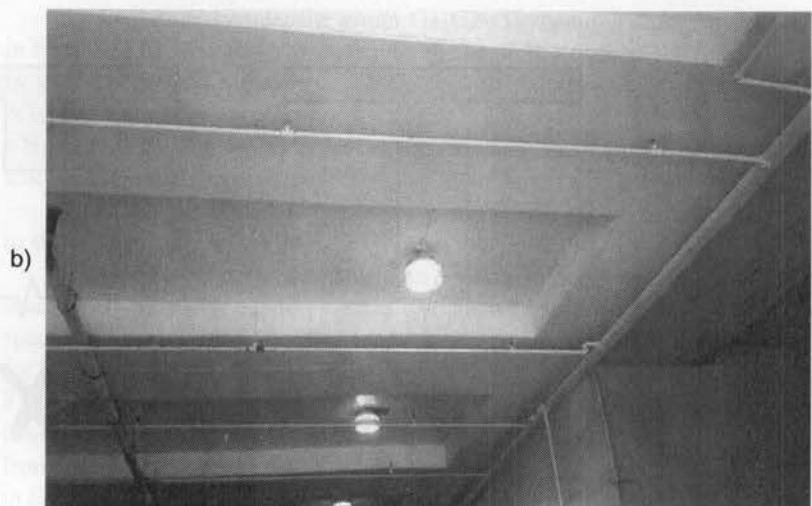
Figure 11.10 Slab band floor system: a) typical plan; b) example of an actual structure.
