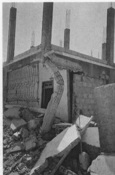
Figure 8.33 Buckling failure of a reinforced concrete column in the 2003 Boumerdes (Algeria) earthquake.
