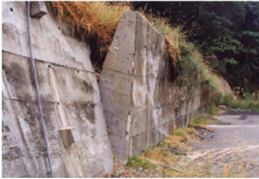
FIG. 2. Trapezoidal concrete gravity retaining wall which rotated outward due to failure of the slope above during the 1999 Chi-Chi earthquake in Taiwan (N. Sitar photo).
