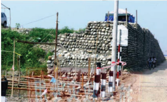
FIG. 3. Cobblestone gravity retaining wall for an overpass, Mianzhu City, China, 2008 (N. Sitar photo).
