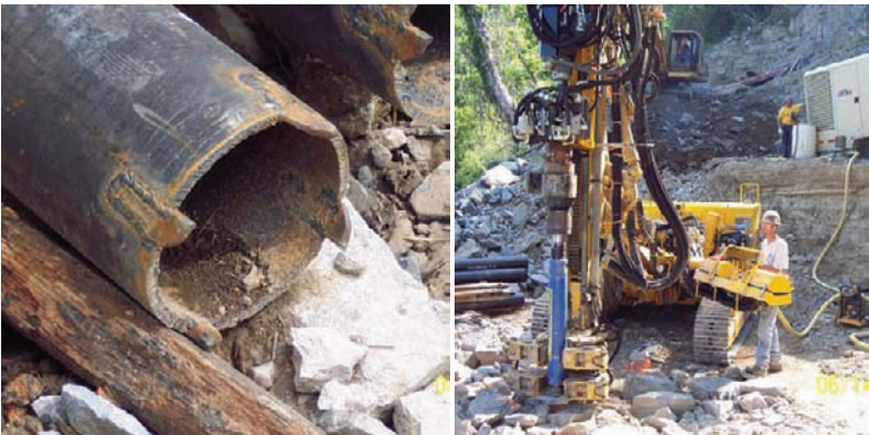
FIG. 3. Micropiles Cased Through Boulder Fill for the Cumberland River Pedestrian Bridge, Nashville, TN.
