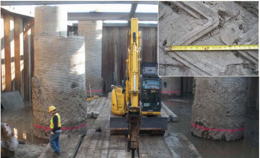
FIG. 13. Exposed Texture on the Drilled Shaft Surface, Huey P. Long Bridge.
