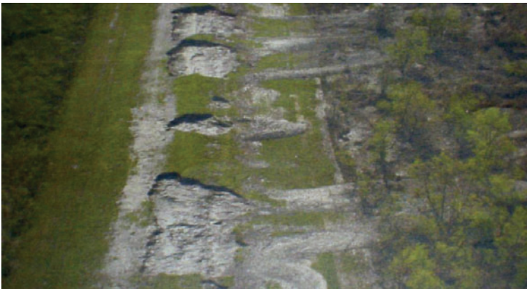
Fig. 3: Partially Eroded Levee Section on the Lake Borgne Frontage (Seed et al., 2008a)
