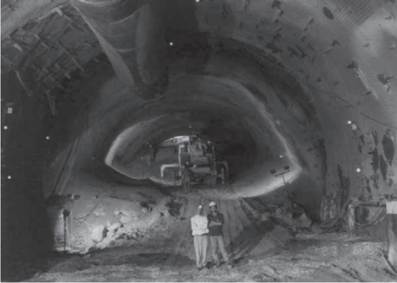
FIG. 11. Bolu tunnel. Heave in the Elmalık right tube at km 54 + 135 constructed per the original design by Geoconsult (1996). After Dalgıç (2002).
