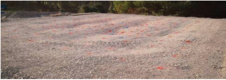
FIG. 11. Differential settlement of CSE Test #5 after dissolving geofoam and applying traffic load.
