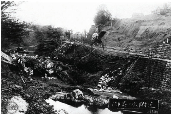
FIG. 1. Failed retaining walls caused by the Great Kanto earthquake (courtesy of the Sykes Kanto Collection, NISEE, UC Berkeley).
