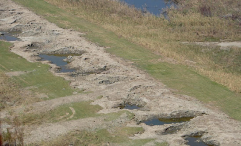
Fig. 2: Erosional Failure on the Lake Borgne Frontage (Seed et al., 2008a)
