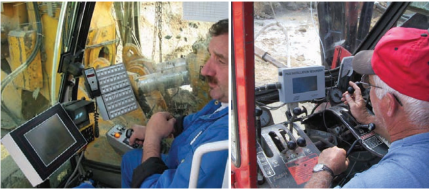
a) Controls on a hydraulic system
