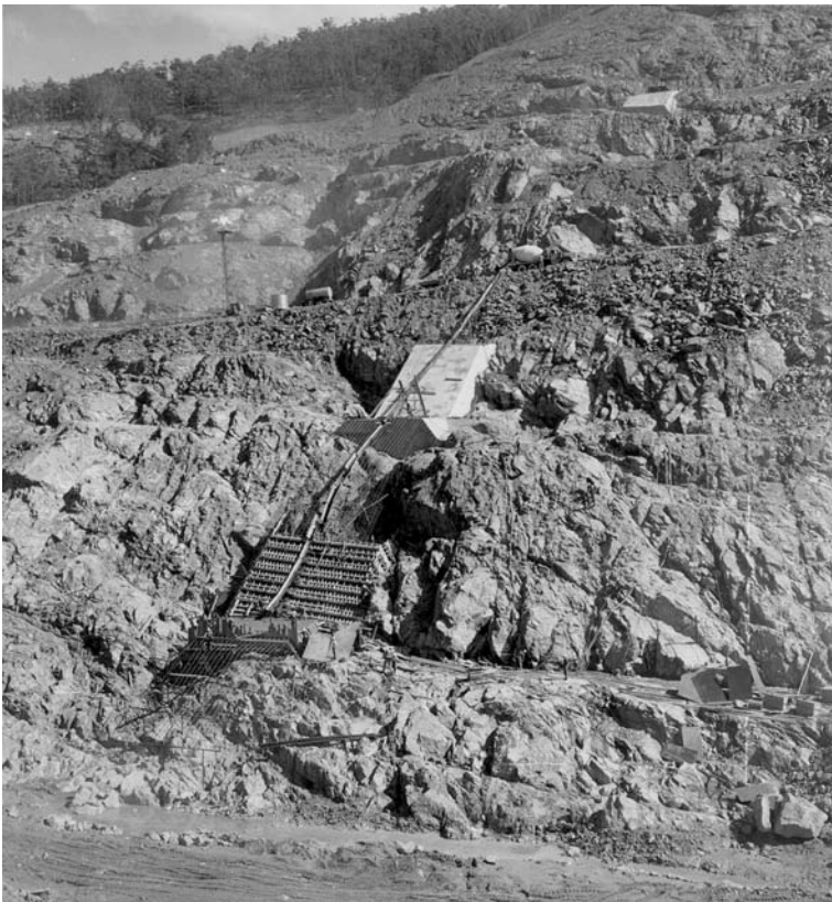
Figure 17.3. Abutment of Dartmouth Dam showing cleanup in cutoff foundation, and construction of the grout cap (Courtesy of Murray-Darling Basin Commission and Goulburn-Murray Water).
