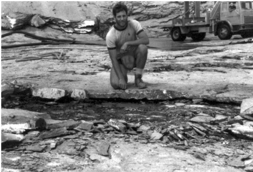
Figure 17.26. Slab of rock which has lifted about 50 mm due to stress relief. Monolith LHZ adjoint to LH1. (Photo courtesy of Sun Water).
