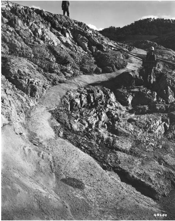
Figure 17.8. Left abutment of Blowering Dam after treatment of large fault zone and weathered seam (Courtesy of Snowy Hydro).
