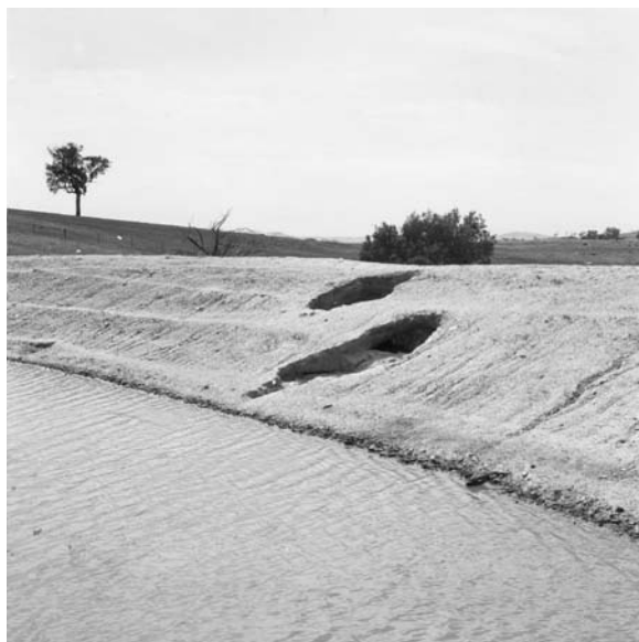
Figure 7.1. Examples of piping failure of a dam due to the presence of dispersive soils (Soil Conservation Service of NSW).
