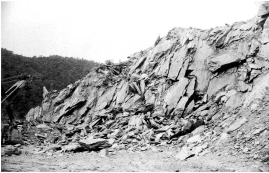
Figure 3.14. Schist being quarried in the spillway excavation at Kangaroo Creek Dam. Note the platy shapes of the rock fragments.
