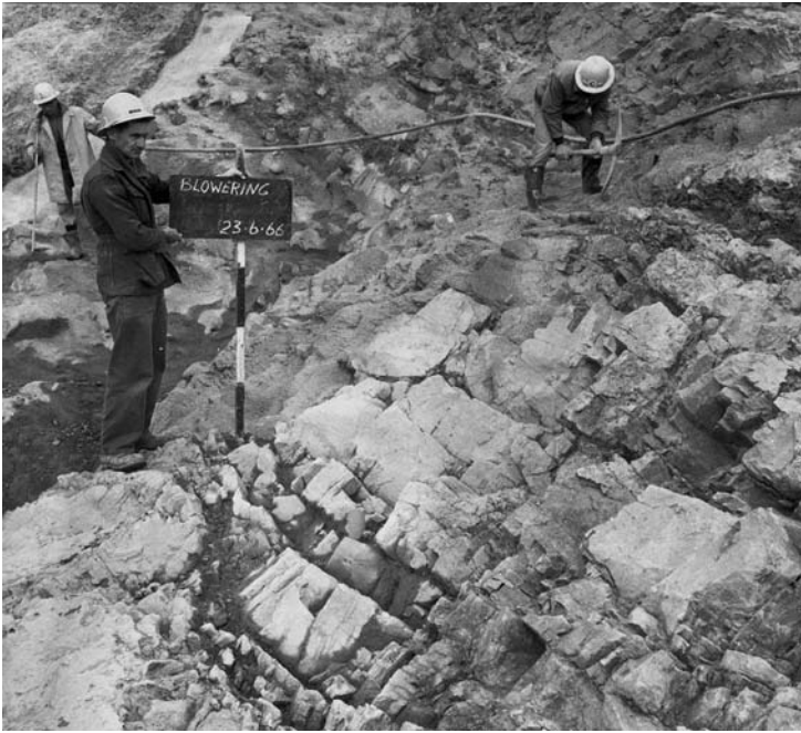
Figure 17.6. Cutoff foundation for Blowering Dam showing open joints being treated with pneumatically applied mortar, but no treatment for other joints (Courtesy of Snowy Hydro).
