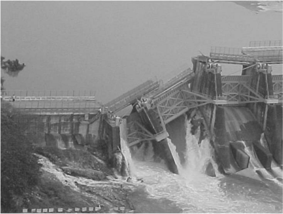
Figure 16.29. Damage to Shikang dam in Taiwan in 1999. The vertical displacement was about 9 m and the horizontal displacement was about 1.5 m into the abutment.
