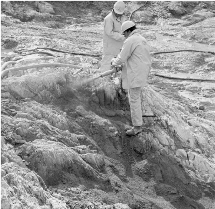
Figure 17.7. Application of pneumatically applied mortar on seams in the cutoff foundation of Blowering Dam (Courtesy of Snowy Hydro).
