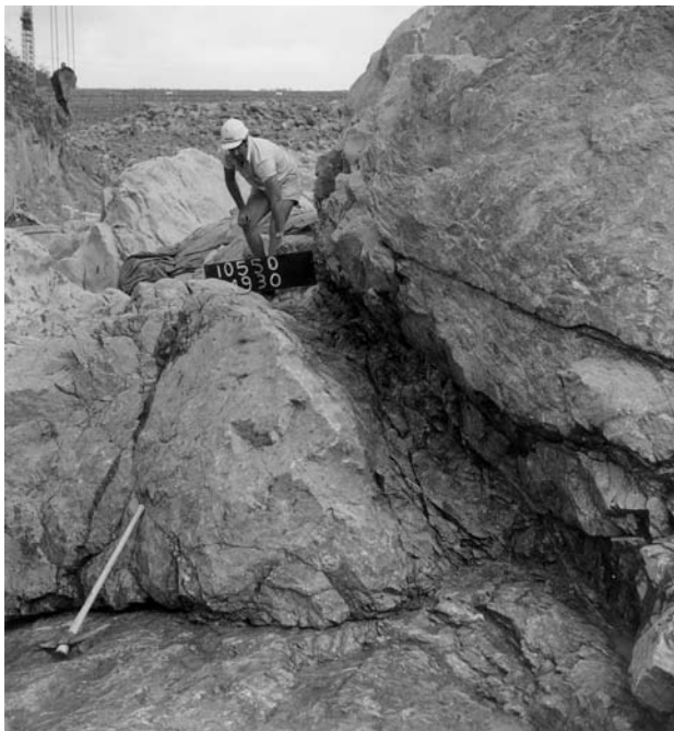
Figure 17.5. Excavation of sheared zones prior to filling with dental concrete in the cutoff foundation of Dartmouth Dam (Courtesy of Murray-Darling Basin Commission and Goulburn-Murray Water).
