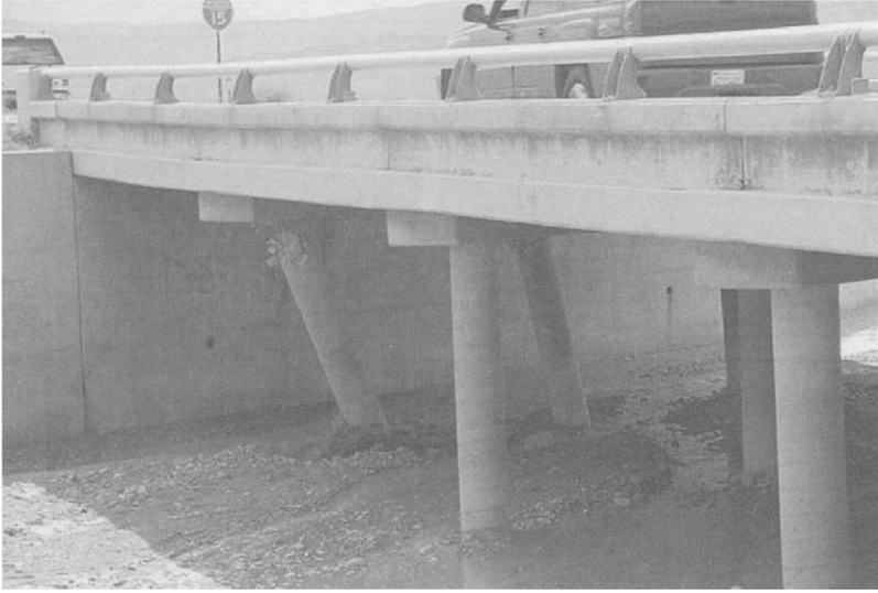
Figure 3.7 Pier failure due to scour. (Source: http://www.dot.ca.gov/ )
