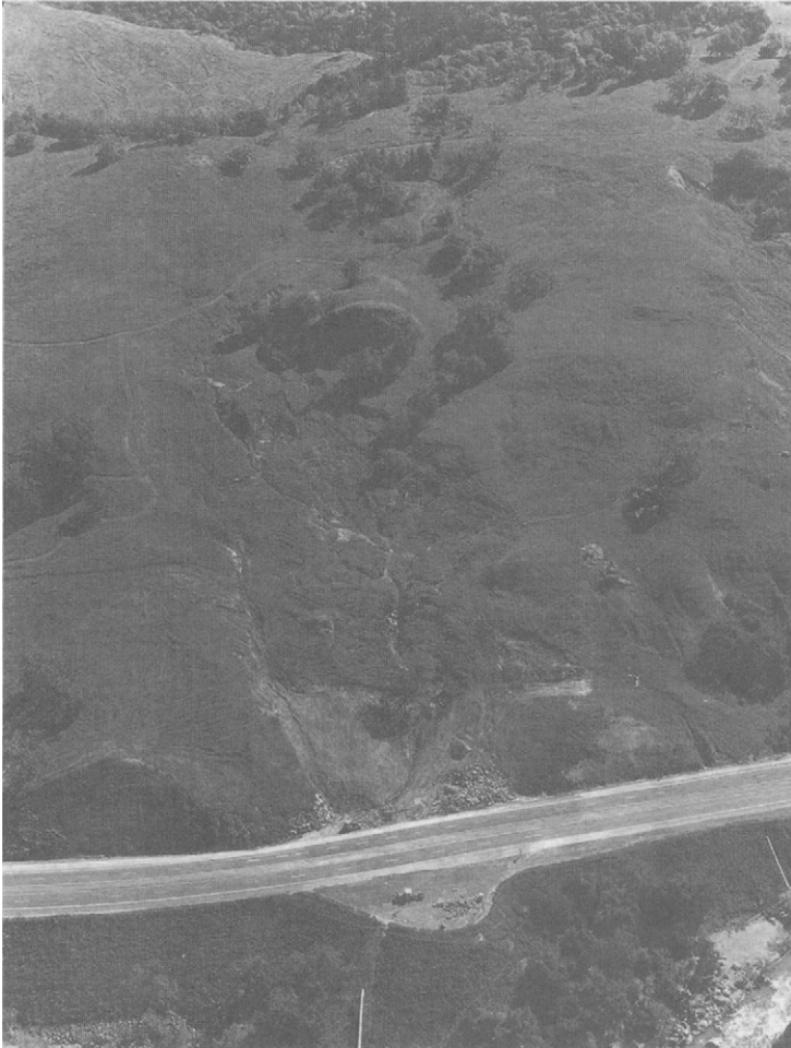
Figure 1.41 Slope failure (Source: http://www.dot.ca.gov )
