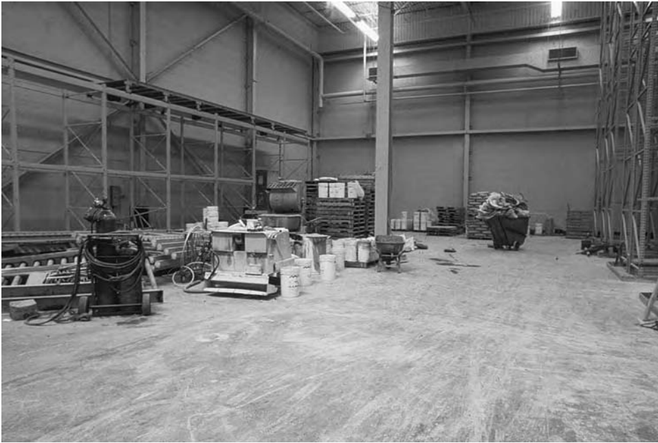
Figure 20.1 Premature wear on an industrial floor
