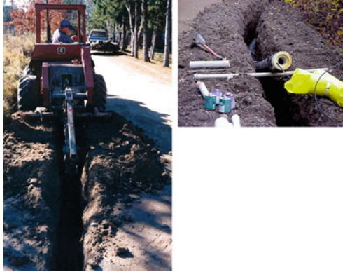
Fig. 5.5 Photographs illustrating the installation of a septic tank effluent pressure sewer (STEP) in a rural development area. Installation is made using a continuous trencher ( left ) and insulation can be added for shallow burial in cold climates ( top ). (Photographs courtesy of R.J. Otis)
