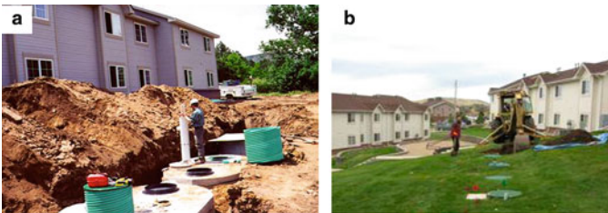
Fig. 6.13 Installation of two 2000 gal pre-cast concrete tanks in series to serve an apartment building: (a) is a view west during installation and (b) is a view east after installation. Note: the risers and secured lids at the ground surface following backfilling
