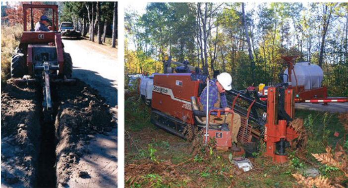
Fig. 5.25 Photographs of effluent sewer main installation using a continuous trencher ( left ) and directional drilling ( right ) methods. (Photographs courtesy of R. J. Otis)
