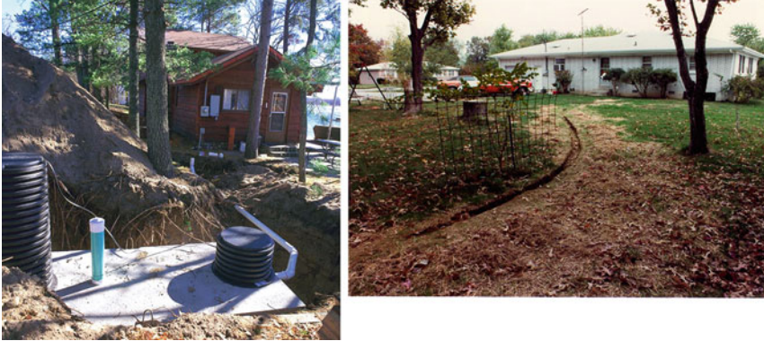
Fig. 5.26 Photographs of a septic tank/pump vault installation along a lakeshore development ( left ) and a service lateral run from a residence to the main sewer line ( right ). (Photographs courtesy of R. J. Otis)
