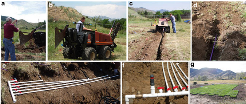
Fig. 12.23 Photographs taken during installation of a drip dispersal unit showing: (a–c) the installation machinery, (d) the tubing placed in a narrow shallow trench, (e) a supply manifold with lateral shutoff valves, (f) a return manifold with shutoff valves and a check valve and air release valve, and (g) placement of Kentucky Bluegrass
