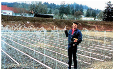
Fig. 8.30 Photograph illustrating the uniform distribution achieved using a pressure distribution network for a RSF that has 1/8-in. diameter orifices designed for discharge with a residual head of 5 ft (Photograph courtesy of Orenco Systems ® Inc.). (The orifices are oriented in an upward direction and will be covered with orifice shields before a layer of fine gravel is placed over the distribution network. The RSF serves 170 EDUs in Elkton, Oregon and is divided into four zones and each zone is pressurized by a 1-hp pump.)
