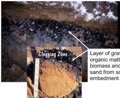
a. Gravel removed from a soil absorption system that has hydraulically failed.
