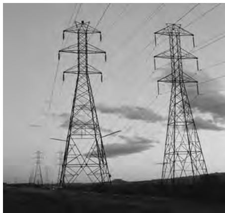
FIGURE 4.26 Electrical power transmission tower and line.
