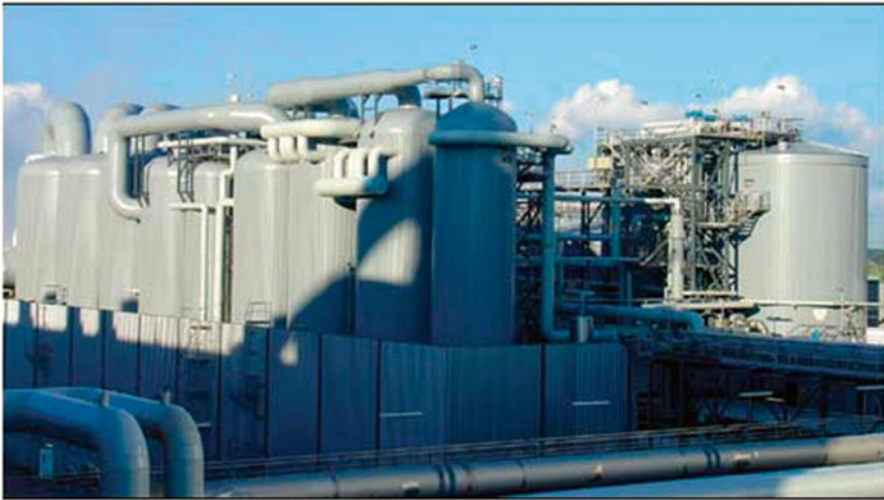
Fig. 5.10 Evaporation plant at Stendal (Toland 2004. Reproduced with permission)
