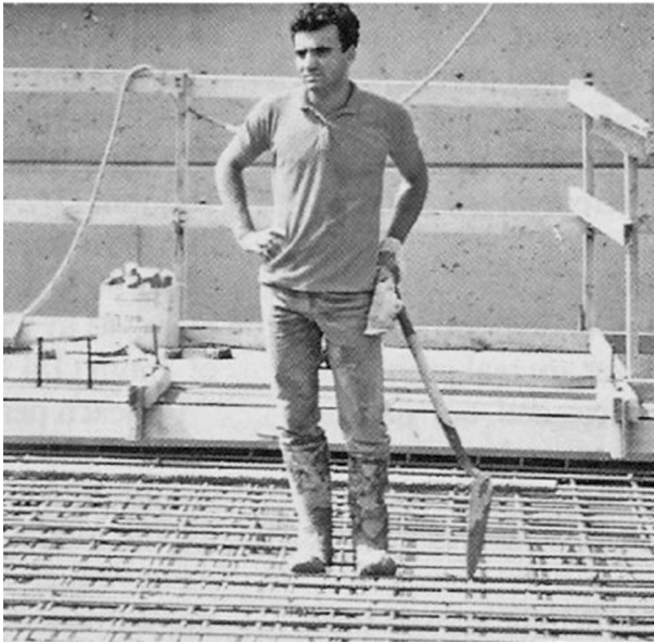
Fig. 6.1.2. Displacement of steel during concreting
