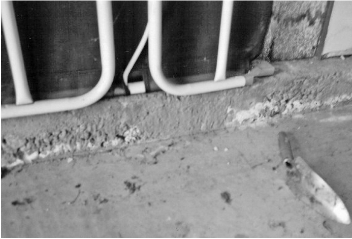
Fig. 4.4.1. Incrustations of salts on the stem wall inside garage. (The stem wall is poorly compacted)
