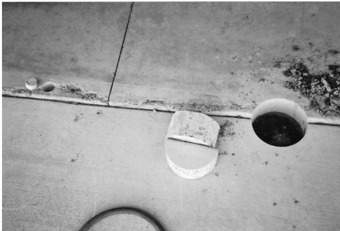
Fig. 4.4.2. Etching of garage floor near entrance from drive. The core shows that the concrete is good
