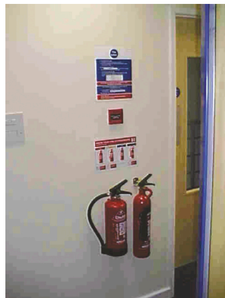
Figure 11.19 Typical fire point in offices with extinguishers, fire notices and alarm break-glass call point
