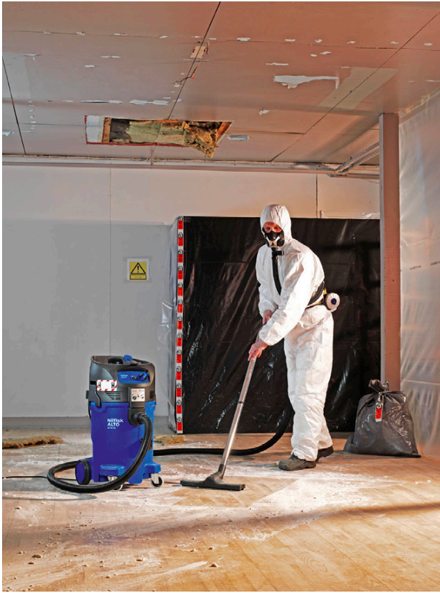
Figure 12.19 High hazard vacuum cleaner to clear up asbestos material
