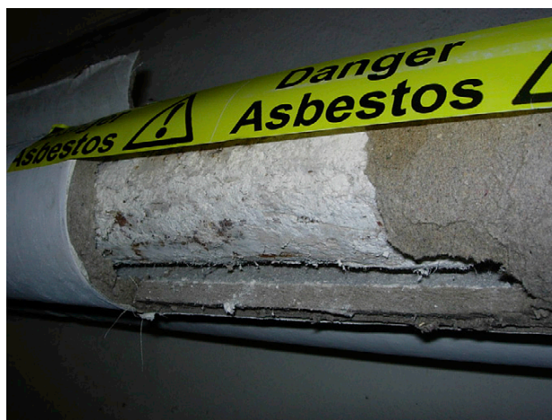
Figure 12.18 Damaged asbestos lagging on pipework
