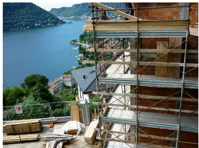
Figure 14.11 Barriers to prevent unauthorized access and handrails to open side of site
