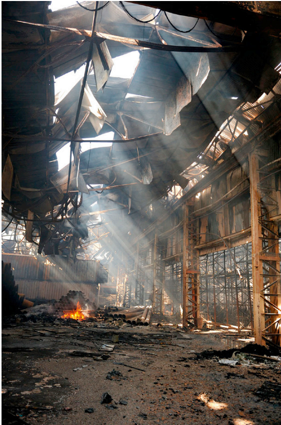
Figure 5.4 A dangerous occurrence – fire
