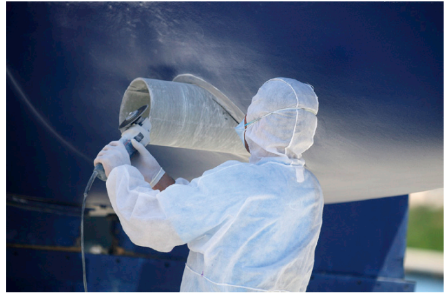
Figure 4.10 A lone worker – special arrangements required
