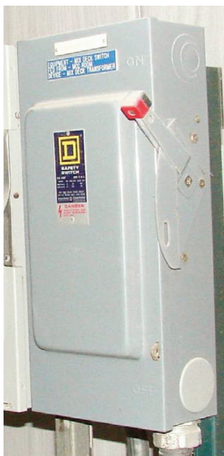
(c) Lockable electrical cabinets.
