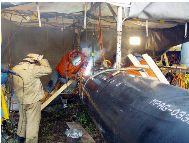
Figure 4.29 A hot work permit is usually essential for welding, cutting and burning except in designated areas like a welding shop
