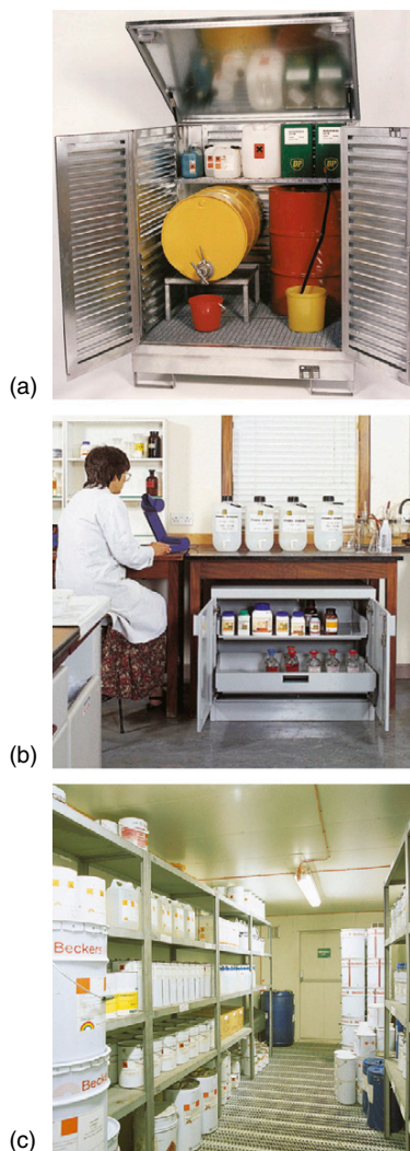
Figure 11.14 Various storage arrangements for highly flammable liquids
