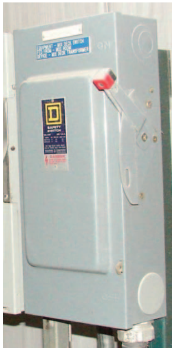
(c) Lockable electrical cabinets.
