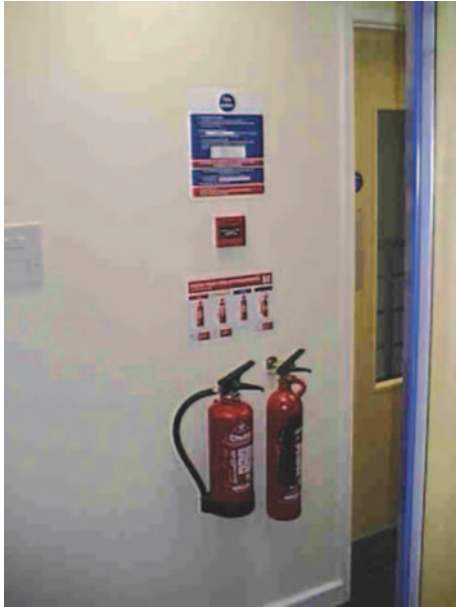
Figure 13.10 Typical fire point in offices with extinguishers, fire notice and alarm break-glass call point.
