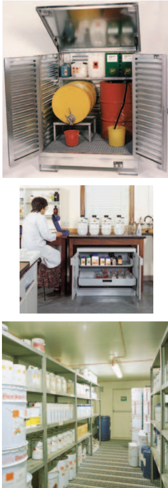
Figure 13.9 Various storage arrangements for highly flammable liquids.
