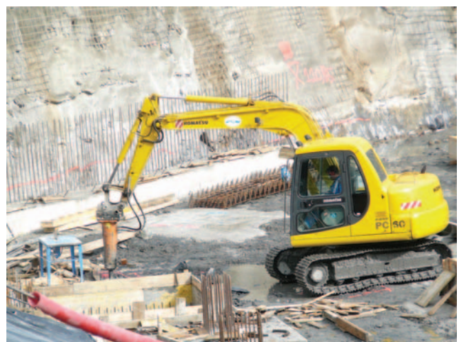
Figure 15.4 Mounted breaker to reduce vibrations.
