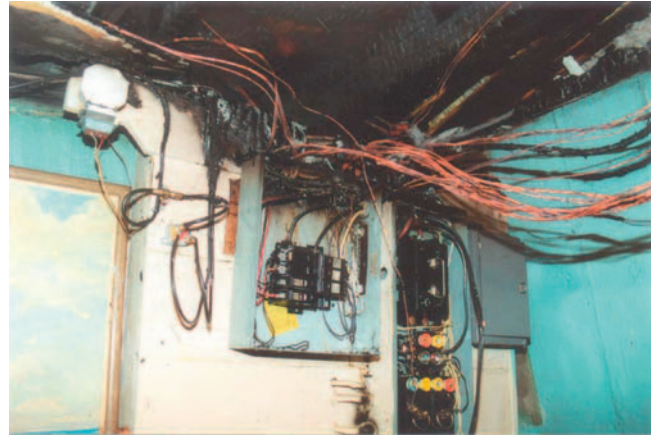
Figure 12.4 Over 25% of fires are caused by electrical malfunction.
