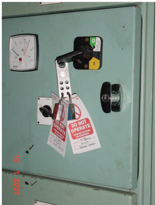
(d) Electrical cabinet with multihasp and lock off padlocks.
