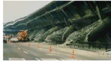
Figure 2. Hanshin viaduct, overturned in Kobe earthquake.
