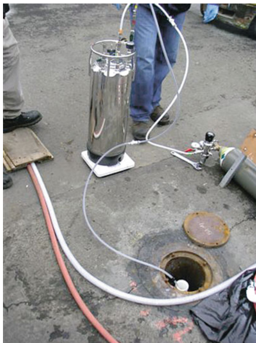
Figure 5.1. Photo of injection of bioaugmentation culture in injection well.
