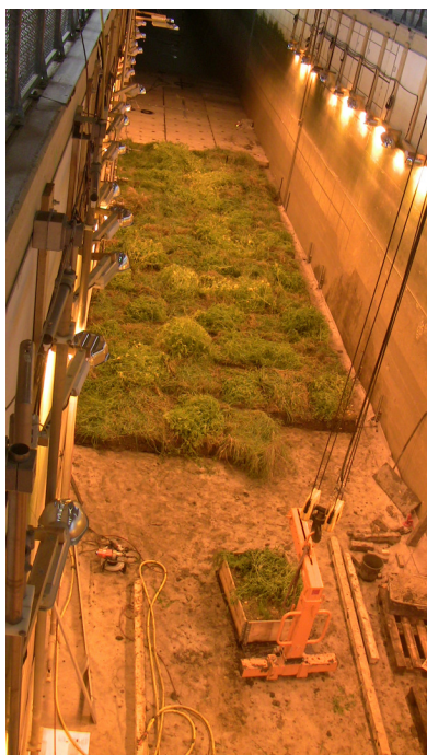
Building a saltmarsh in the Large Wave Flume (Grosser Wellenkanal, GWK) of Forschungszentrum Küste (FZK) in Hannover, Germany, to test over-marsh wave energy dissipation under storm waves. The flume is 330 m long, 7 m deep and 5 m wide. Photograph by Tom Spencer.
