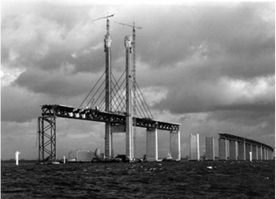
Figure 7-9. GPS/RTK technology was used in the construction of the Øresund Bridge between Denmark and Sweden.
