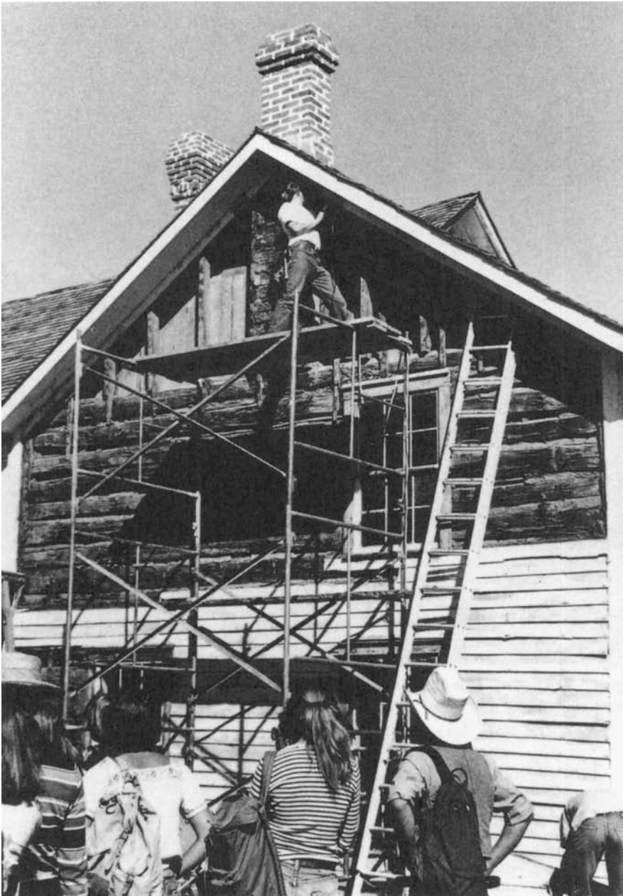
Figure 5.29. The Four Mile House with clapboard siding covering the original walls. Photograph courtesy of Four Mile House Historical Park.
