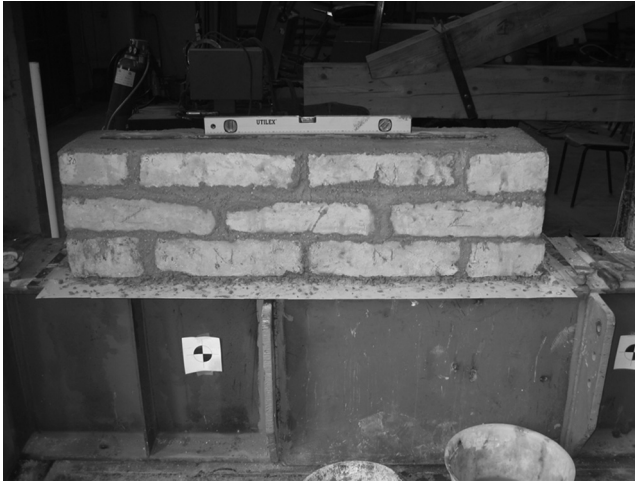
Figure 16.4 An adobe wall under construction made by rectangular blocks arranged next to one another and put with alternate earth mortar joints.
