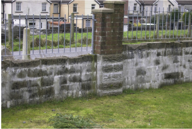
Figure 18.1 Discoloration (efflorescence) of a masonry wall caused by excessive lime or other salts in the materials used.
