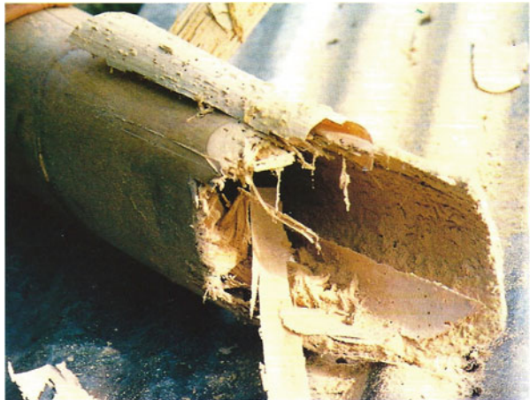
Fig. 9.10 Culm deterioration by termites (Liese and Kumar 2003)
